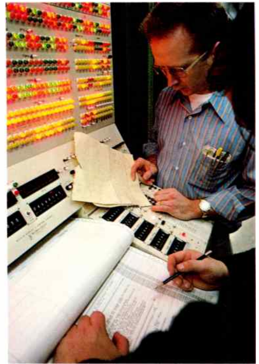
Sophisticated telecommunications equipment displays status of central processing unit at the Lena Point, Alaska, switching center.
