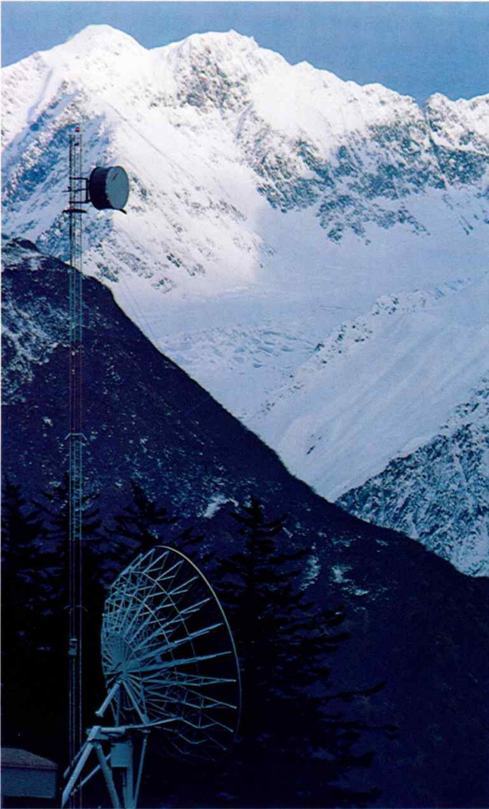
This Alascom satellite earth station is located at Valdez, the southern terminal of the trans-Alaska oil pipeline route.
