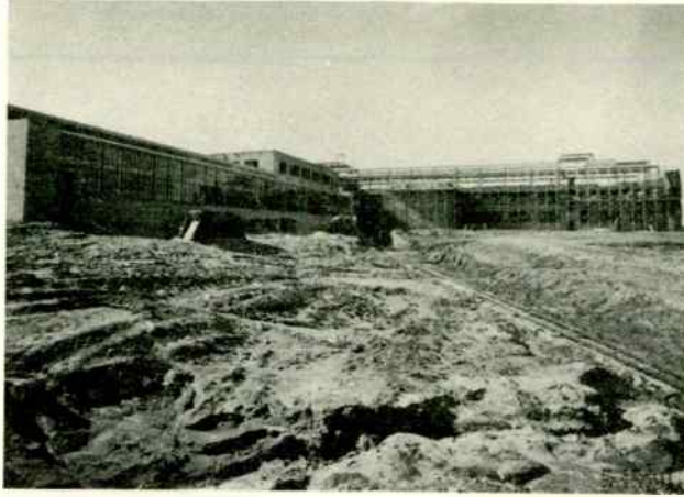
VIEW LOOKING NORTHWEST SHOWING PROGRESS ON BRICK WORK OF EAST WING AND COMPLETION OF GLAZING ON REAR BUILDING
