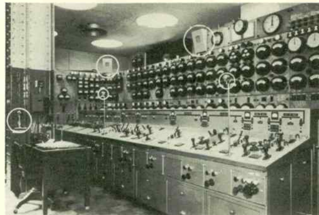
CONTROL ROOM - PHILADELPHIA ELECTRIC COMPANY - SHOWING MICROPHONES AND LOUD SPEAKERS
