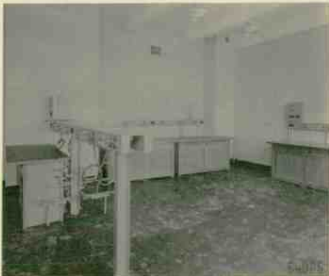
One of the Laboratory Rooms with Bench and Power Installations Partially Completed
