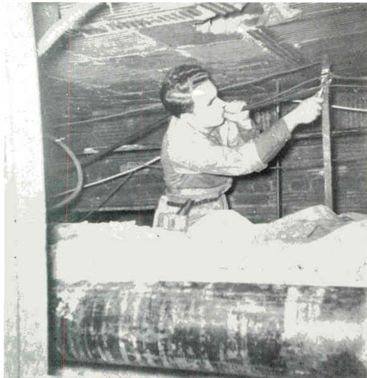
North Pittsburgh's Dick Moore working "in the shafts" of the Hotel William Penn on some of the more than 10 miles of cable used in the huge job
