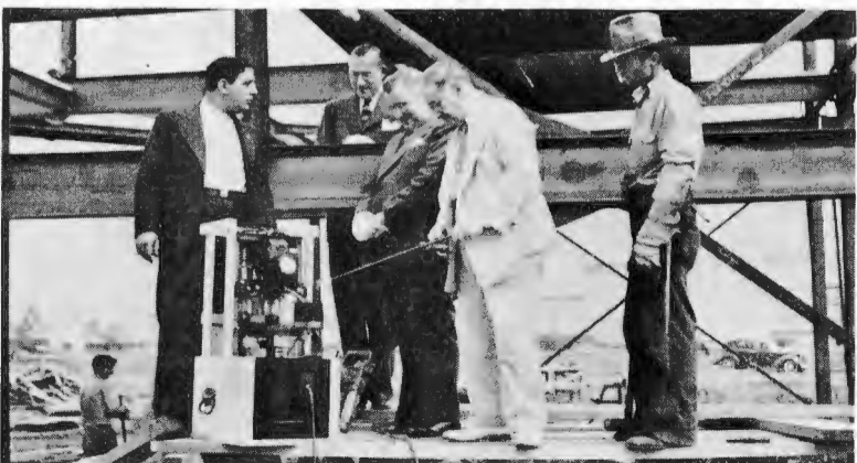
Radio waves were used to heat the last rivet as steel work on the Radio Corporation of America's exhibit building in the New York World's Fair 1939 was completed. Participating in the event were, left to right, Joseph D'Agostino, RCA exhibit co-ordinator; H. C. Bonfig, commercial vice president of RCA Manufacturing Company; Robert Shannon, vice president and general manager of the same company, and John de J. Almonte, assistant to the president of the National Broadcasting Company
