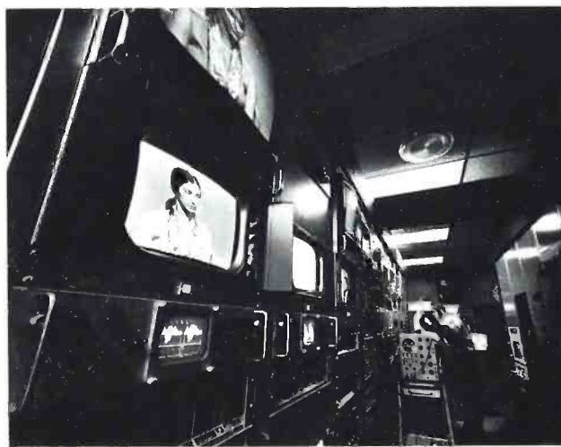
RCA continued to be the leading supplier to the broadcast industry. This RCA broadcast equipment is installed in a new UHF station in Trenton, N.J.
