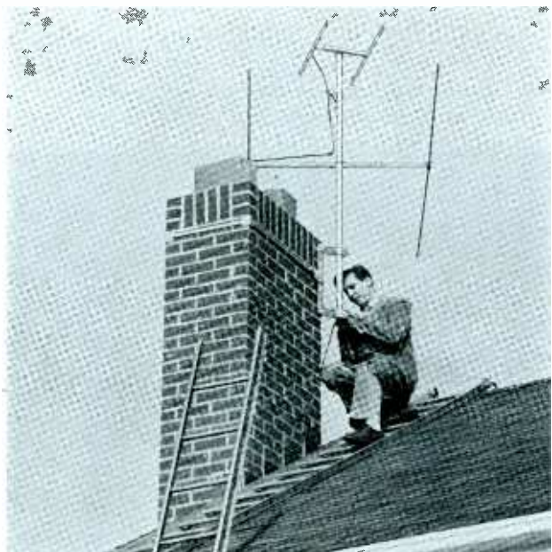
Technician of the RCA Service Company installs an antenna for the owner of an RCA television receiver.
