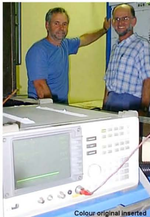
Will (on the left) and fellow worker Ian with the Dili TV transmitter. The spectrum analyser in the foreground shows how clean the signal is
