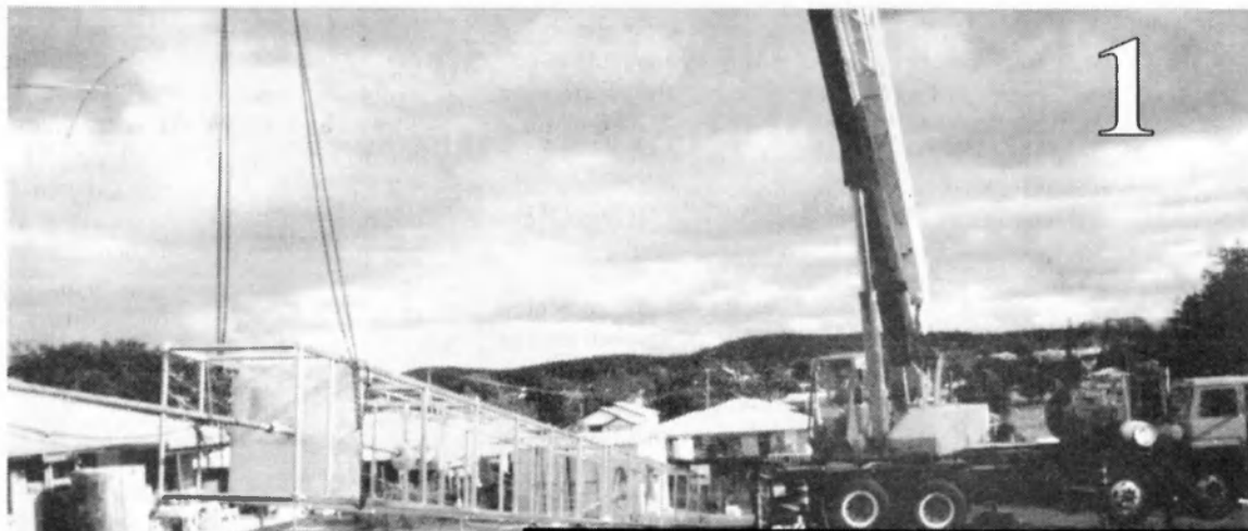
News tower on the ground, about to be hoisted into position by a hired crane
