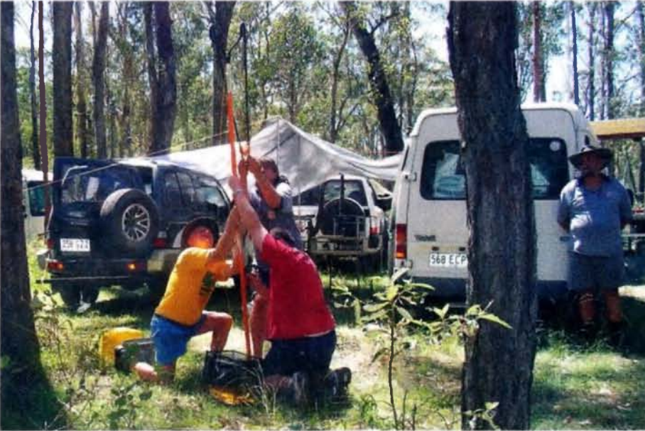
George, Peter and Shaun get the wires over the trees while Kerrod watches from a safe distance.
