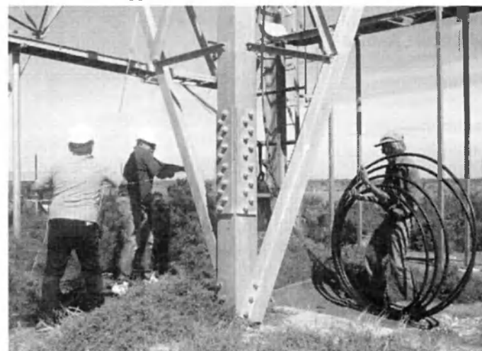
Figure 1 l to r. New member Paul, Club Secretary Paul Gale VK5ZKG and John Ross VK5NI hauling one of the two LDF5-50 coaxes to the top of the tower. The workers also give some scale to the structure
