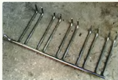
Photo 2: Cable rack bent.
