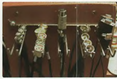
Photo 3: Cable rack with cables.
