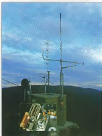
This month's cover The main photo shows the VK7RML repeater site on Mt Lloyd, quite a remote location. See the VK7 News column for an update on this repeater. Photo by Hayden Honeywood VK7HA. Inset photo shows some of the internals of the homebrew 160 m AM transmitter built by Noel Ferguson VK3FI. Photo by Noel Ferguson VK3FI.
