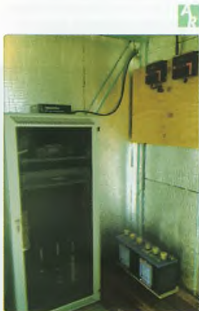
Photo 3: Inside the fully insulated shed are the 'internals' of the CQARA 70 cm repeater. The solar panels produce 400 watts to power the site.
