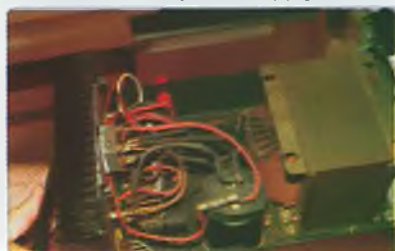
Photo 1: The old power supply.
