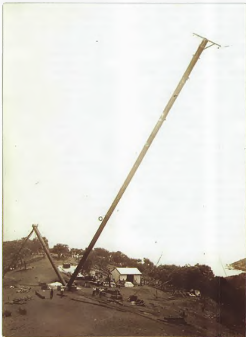
Photo 1: The 60 metre mast on its way to its vertical position. Note the method of erection, via the use of a fulcrum. Printed with permission of the Cooktown Historical Society.
