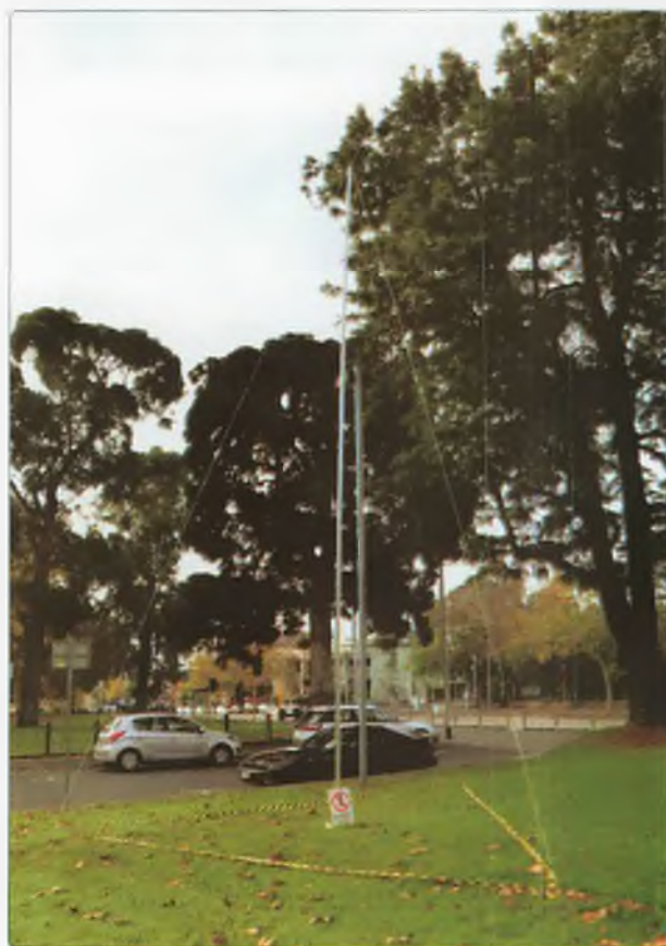
Photo 3: An antenna support mast set up in the gardens. Note the safety signage and warning tape.
