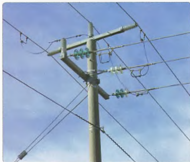
Photo 4: Modern concrete pole and hardware knuckle insulators.
