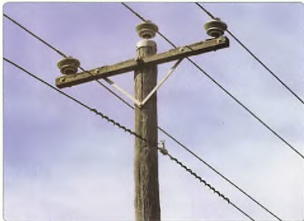
Photo 6: Old timber pole with loose cross arm supports.
