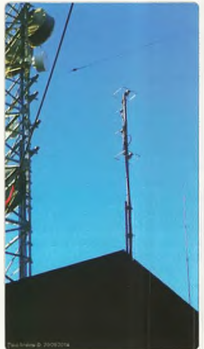
Photo 2: VK2RSY 2 m and 70 cm beacon antennas now installed on the roof of the VK2WI building.
