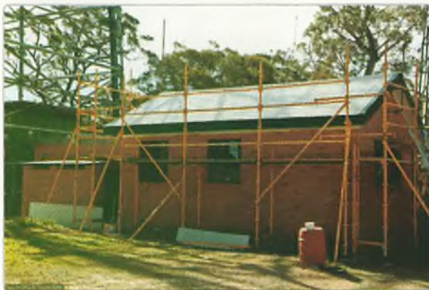
Photo 1: The asbestos removal and fire proofing of the ARNSW VK2WI building is now complete along with a new toilet block.
