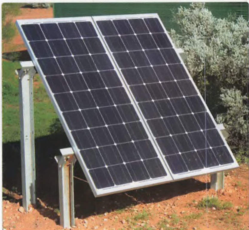
Photo 4: The two solar panels.
