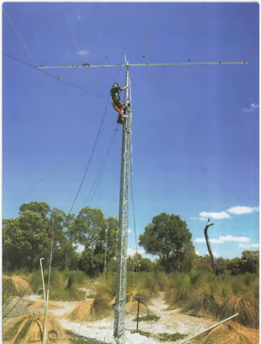
Photo 2: Antenna activity at NCRG. President Stu VK6LSB our licenced rigger at the top of the mast fitting the first of the 15 m modified beams.
