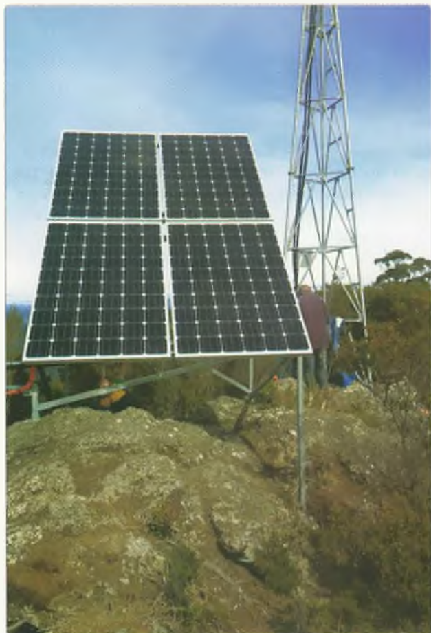
Photo 8: Antenna mounted and solar panels.
