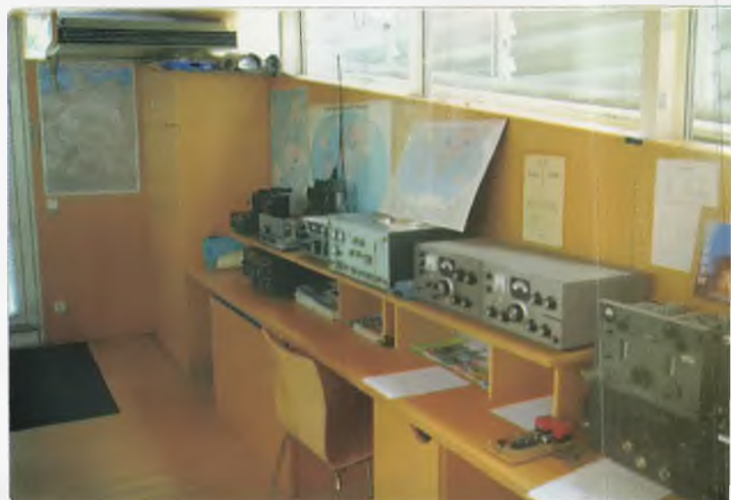
Photo 2: The view through the window of the shack showing one bench of equipment.
