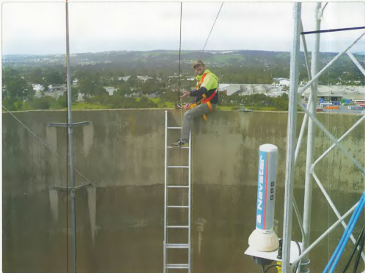
Photo 3: Damien VK5FDEC attaching a guy wire to the rim of the tank over 50 m from the ground. The GPS antenna for the reference is at the lower right.
