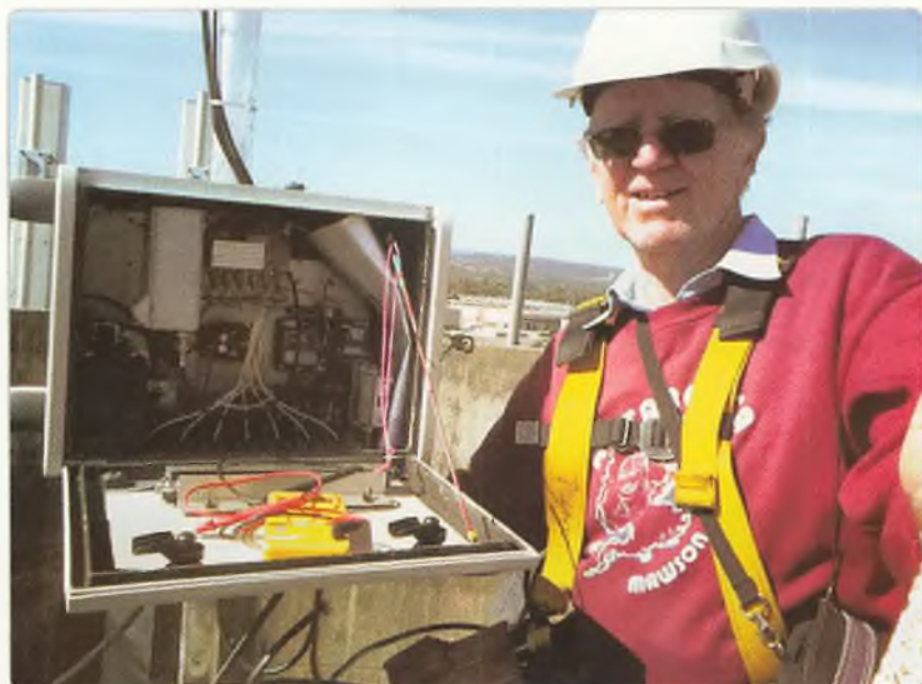
Photo 4: Keith VK5OQ with the reference and DC distribution unit in place on the Water tower.
