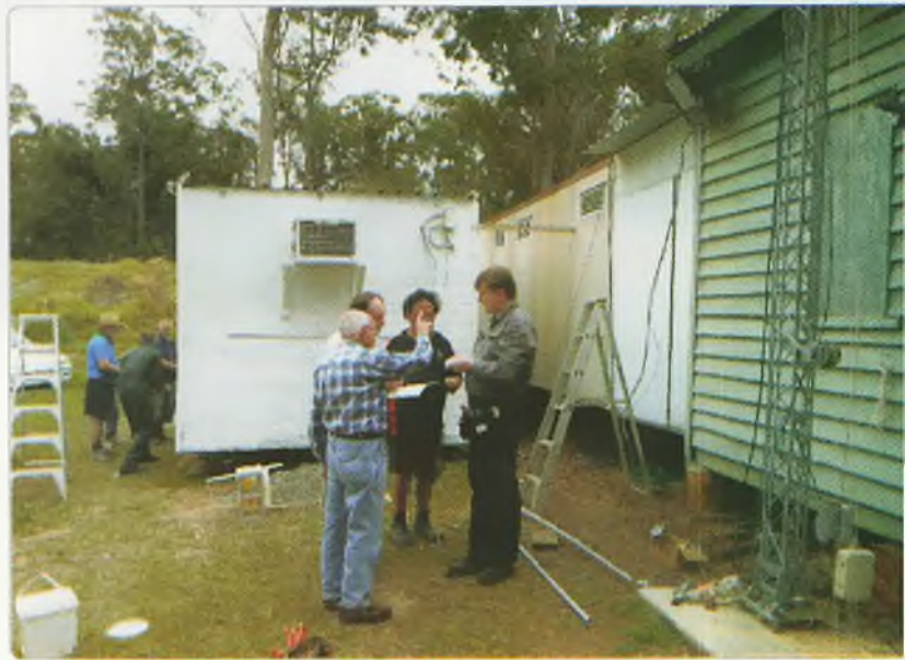
Photo 1: Jim VK4FKGF (hand raised) giving instructions to members on the installation of the mains power cabling.
