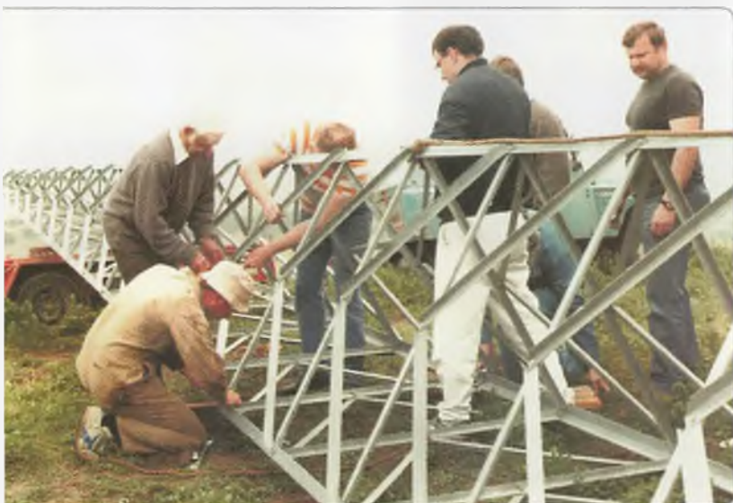
Photo 2: The mast at Mt Anakie.
