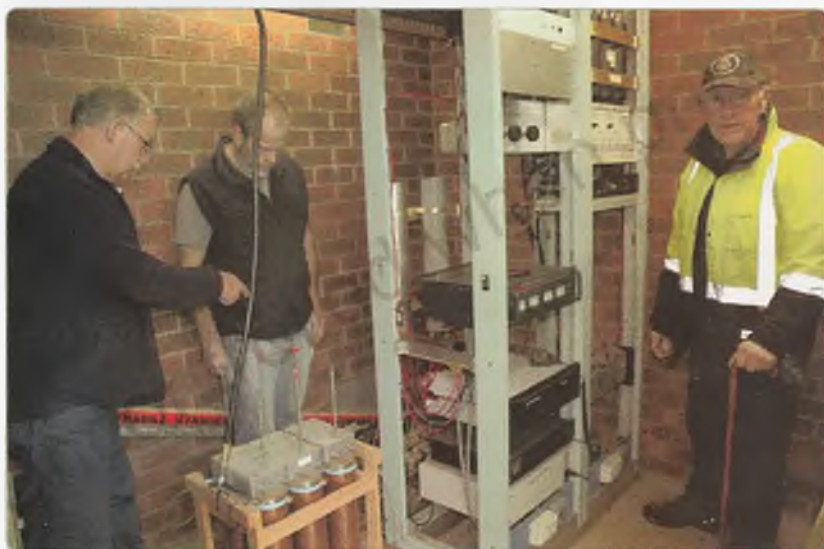
Photo 1: The rack mounted equipment for the 2 m and 70 cm VK3RGL.
