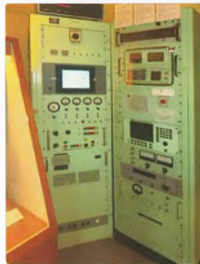
Photo 7: Omega Station Control Racks.
