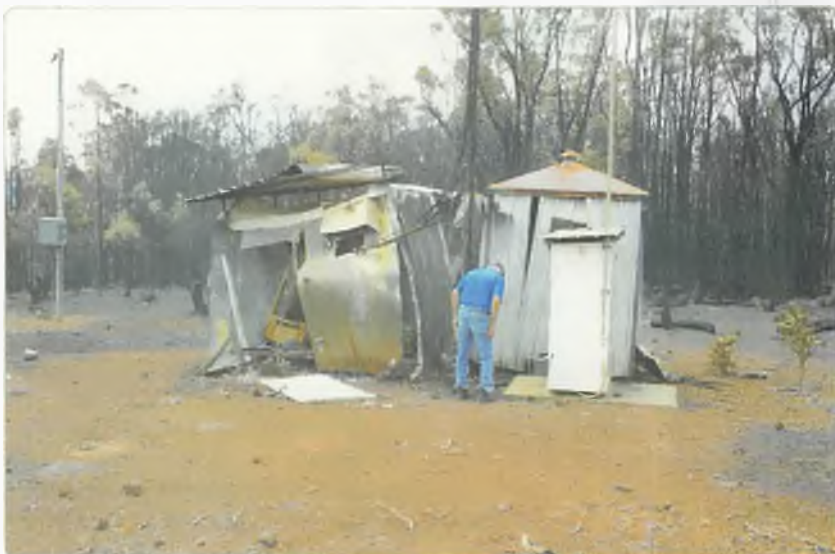
Photo 1: Looking over the area around the VK6RMW equipment shelter after the fire.
