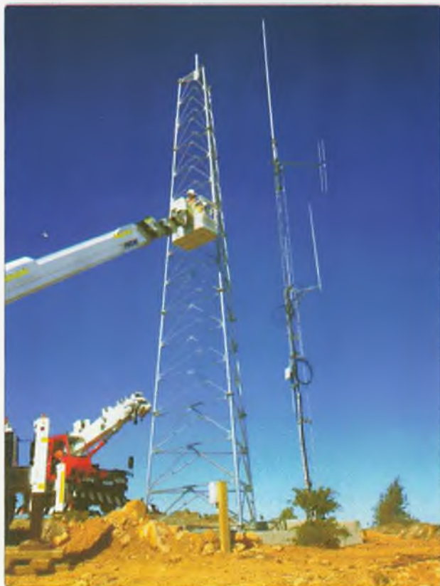
Mt Wombat repeater site new mast to replace old guyed one.
