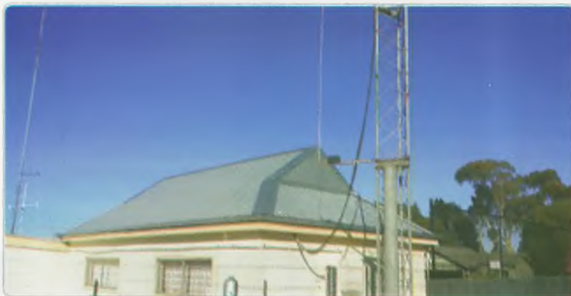
Photo 2: The new roof adjacent to the west tower of the GARC Club house.
