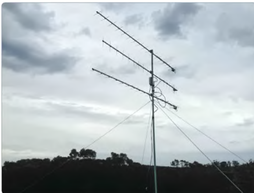
Photo B: 70 cm antennas - 19 element horizontal stack for SSB, 19 element vertical beam for FM mounted on 6 metres rotatable pole.
