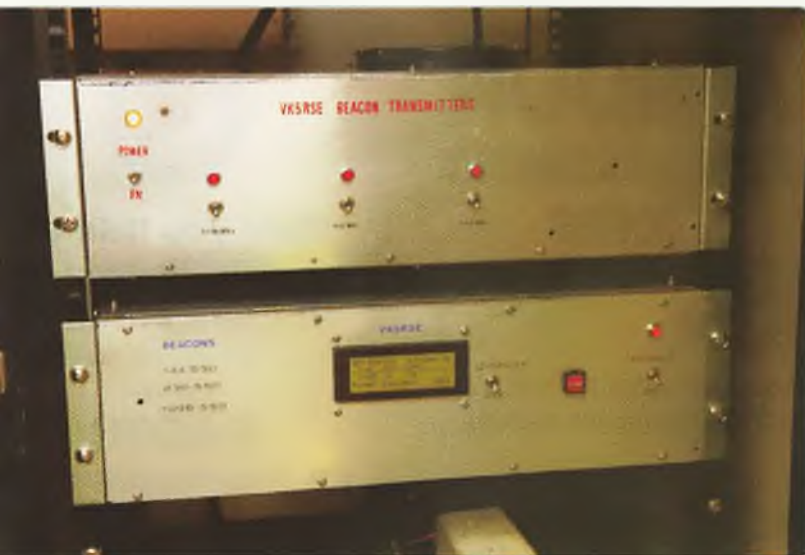
Photo 2: Close-up of the Beacons: Top the final amplifiers and bottom the excitors. The display cycles through time/date, GPS data, TX status, temperature and mode. Just showing is the white remote control receiver in a die cast box.
