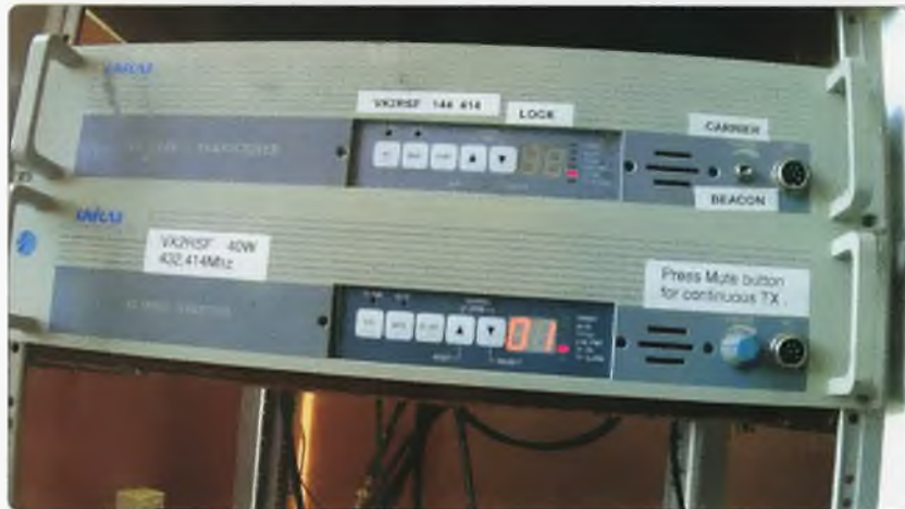
Photo 1: The new beacon transmitters for VK2RSF. Photo by Rod VK2TWR.
