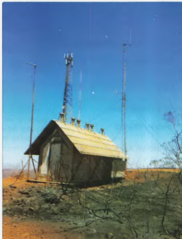
Photo 5: Equipment building and towers after the fire.
