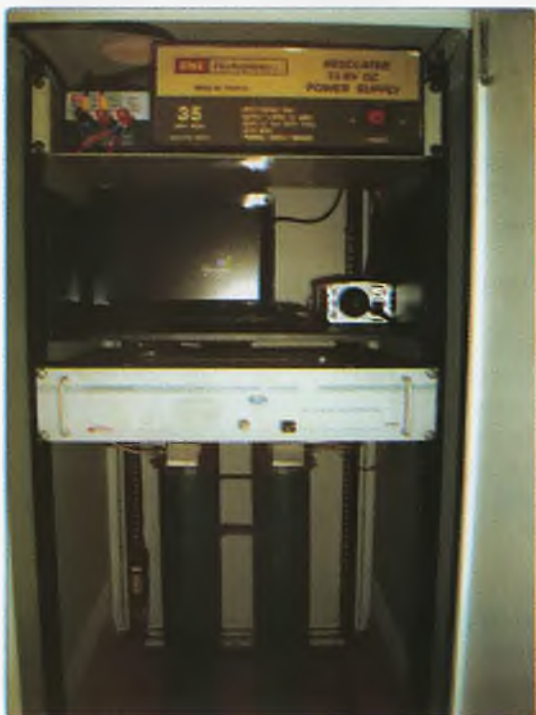
Photo 3: Inside before the fire was the equipment rack.
