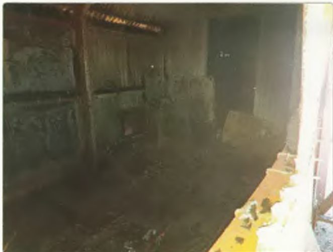
Photo 6: Inside the equipment room after the fire.
