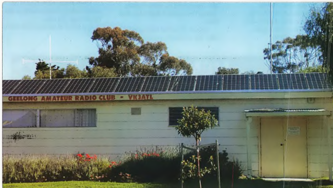
Photo 1: Solar Panels on Club House roof.
