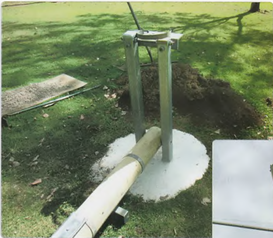
Photo 5: The mast base with the mast ready to elevate to the vertical position.
