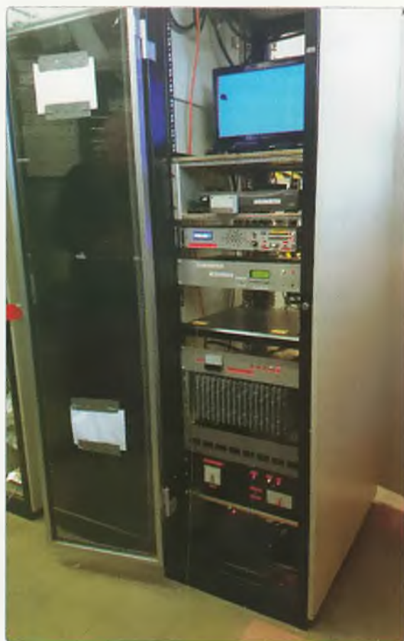
The equipment rack for VK3RTV Surrey Hills.
