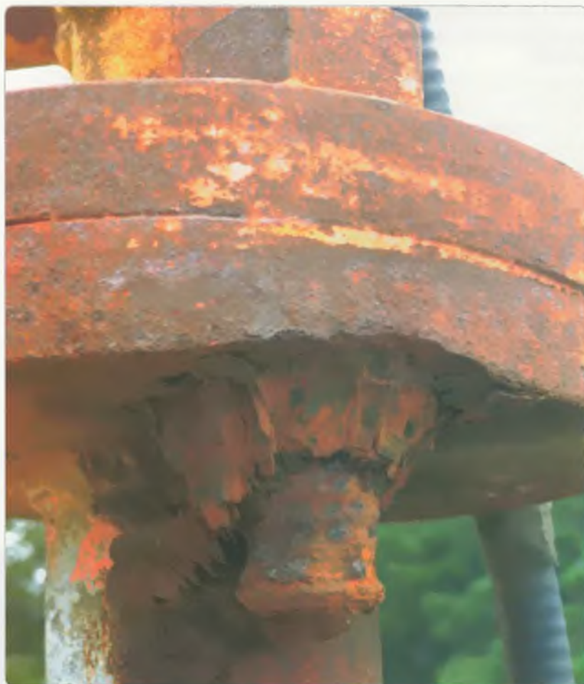
The tower at Crafers showing its very poor condition.
