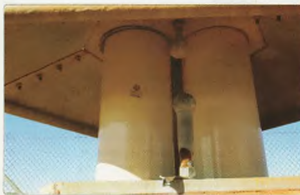
Photo 2: The porcelain insulators at the tower base, together with a spark gap for static discharge and lightning protection.
