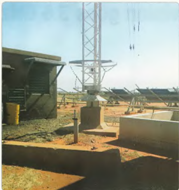
Photo 9: View of the antenna mounting at the De Grey site.
