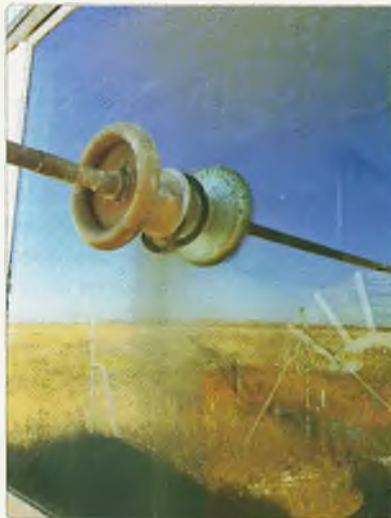
Photo 3: The feeder exiting the transmitter hut.
