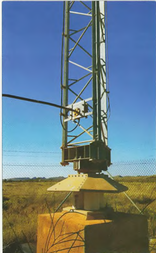
Photo 4: The Woodbrook antenna base and feed arrangement.
