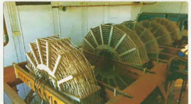
Photo 5: Inside the Woodbrook Coil House showing the impressive tuning coils in their timber mounting rack.
