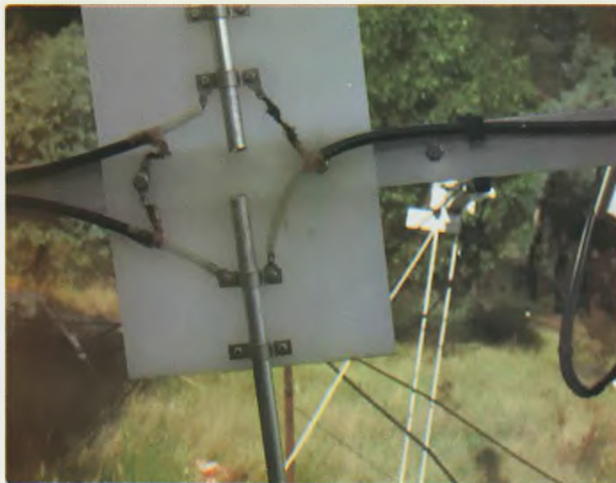
Photo 6: Detail of the mounting and feeding of the driven element.
