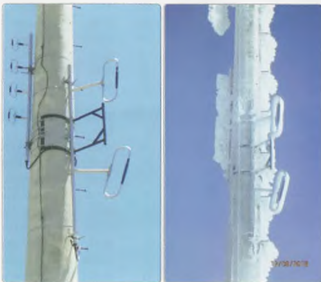
Ice damage to Mt. Hotham APRS antenna.
