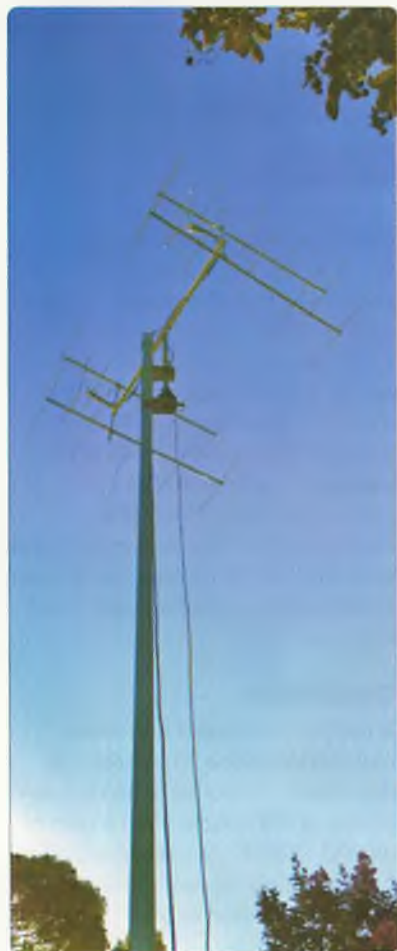
Photo 1: Array on tower.
