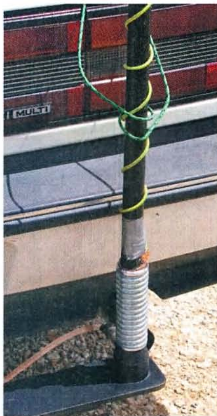
Photo 1: A close up of the antenna mount, showing the end to the tag soldered on to the copper washer.
