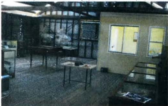
A view of the inside of the shed, all nicely coming together.
