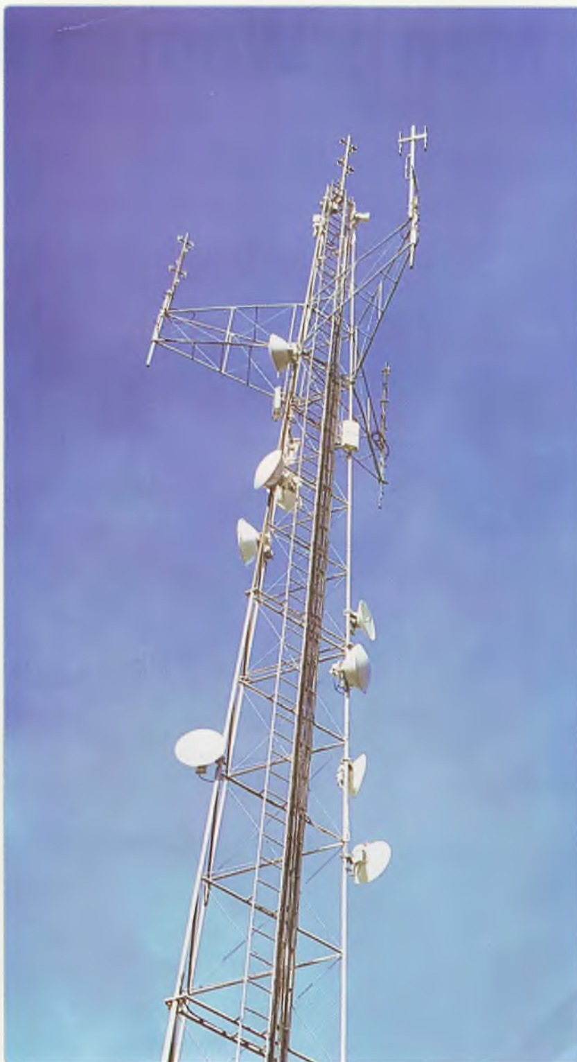
The VK3RTV antennas are high on the tower at Mount View.
