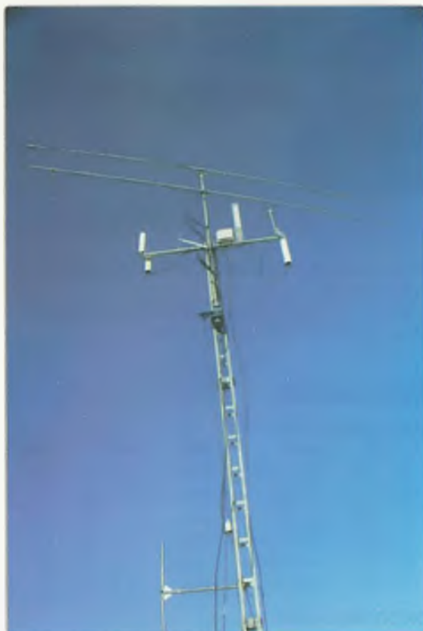
Complete array of antennas located below Rob's 24 m and 70 cm Uda Yagi antennas.
