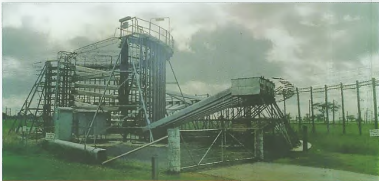
View of the antenna switch matrix that could switch up to 35 antennas and 10 transmitters, including the dummy load.
