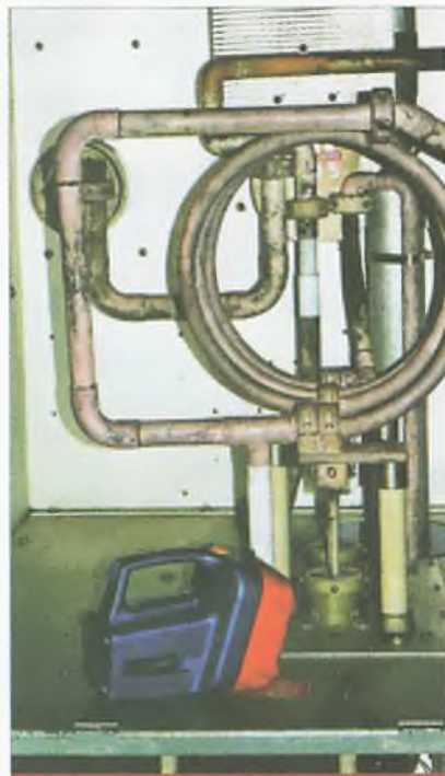
Tank circuit of the final stage of a 100 kW Harris SW100A transmitter. The torch provides size perspective.
