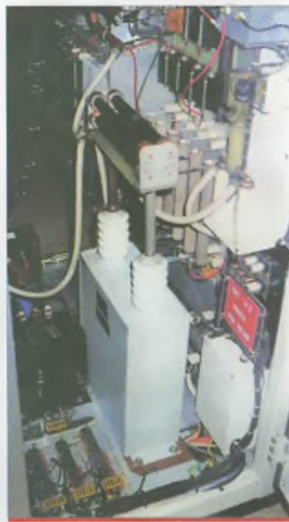
Showing part of the power supply of a Harris SW transmitter.
