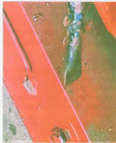
Photo 4. The flattened pipe end, before drilling to take a bolted-on lug for the earth stake link.
