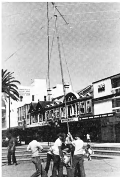
PHOTO 5 The beam mast in a bucket of beach sand, then comes the water to harden the base, which is a plastic garbage bin.
