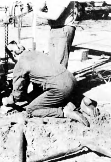
As with all things electronic, there is room for Murphy's Law! Here is Steve VK6YK with assistance from Ross re-arranging the concrete mounting block because it had been put in the wrong way round.
