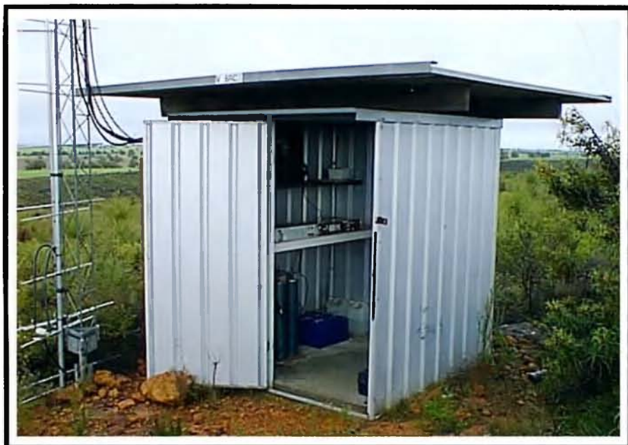
The Cataby repeater site. (Colour original inserted)
