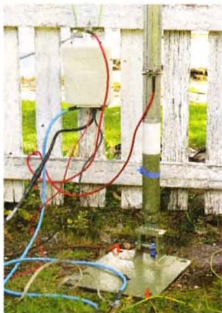
The base loading antenna tuner.
