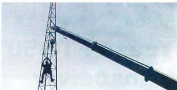
Photo 1: Ian Campbell VK5NIW attaching the crane cable to the tower for lowering.
