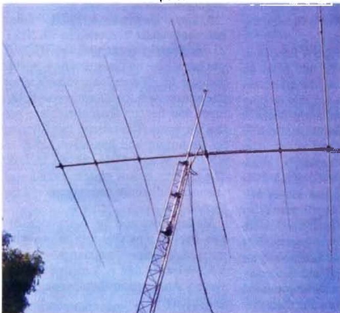
Photo 8: The TH6DXX atop the tower.
