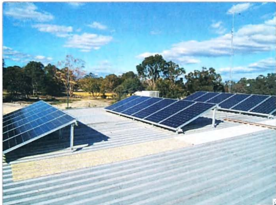
Photo 2: The solar panels on the NCRG clubrooms roof.
