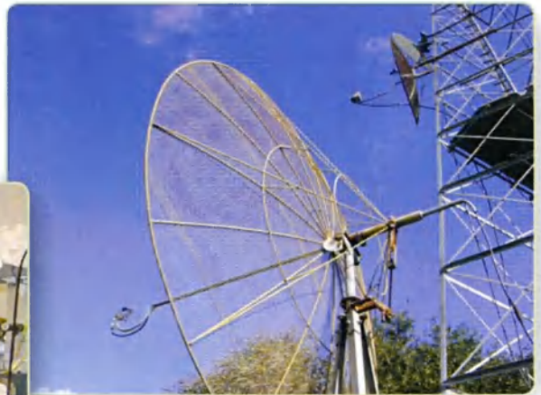
Microwave antennas close up – fixed pointing at Adelaide!
