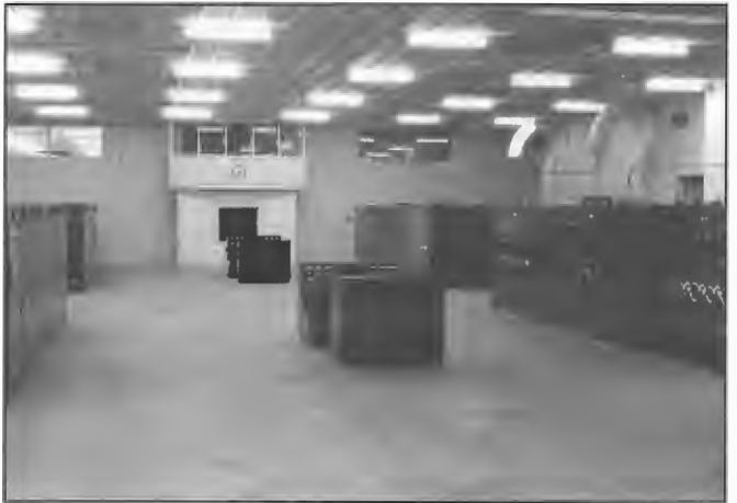
Transmitter Hall, Radio Australia, Shepparton 1946. Left: 10 kW AWA transmitter. Right: STC/AWA 100 kW transmitters high power stages. Centre: Control and aerial switching desks. Alan McIntosh was the first Resident Engineer.
