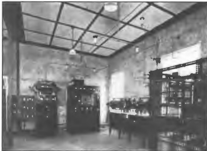
AWA 5 kW transmitter commissioned for 4QG Brisbane in Queensland State Insurance Building 22 April 1926. It was similar to AWA transmitters installed for A Class stations in other States at the time. Chief Engineer-in-Charge of operations was Fred Stevens.
