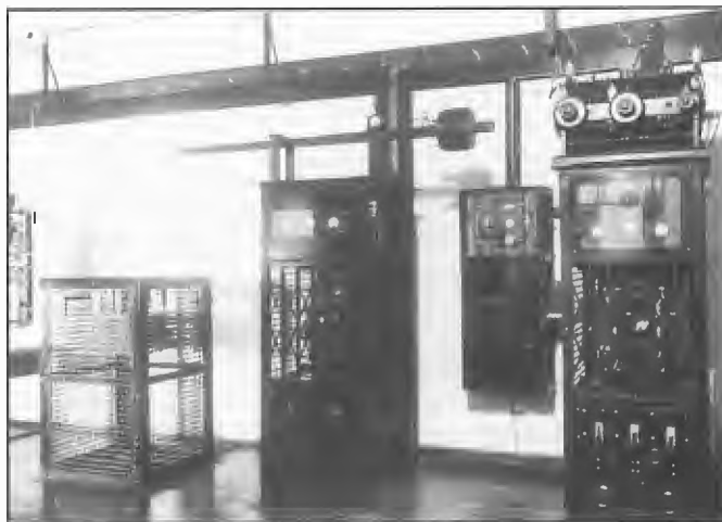
Other sections of the 6WF transmitter. The total installation comprised three phase HT supply, power amplifier and modulator, submodulator and line amplifier, master oscillator, closed circuit inductor and capacitor and the aerial circuit inductor.
