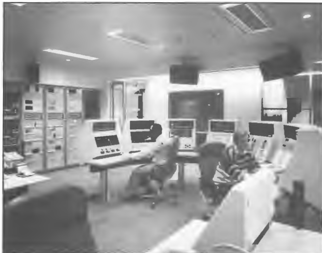
Master Control is the technological heart of the ABC Ultimo Centre, Sydney. It manages the switching of the same program to a number of ABC Radio stations across Australia; program source selection, whereby a studio in Sydney is linked with another studio for long-distance interviews; quality control with responsibility for ensuring broadcast quality at all times; and network integrity to ensure that each network or station remains on air at all times. (Courtesy ABC.)
