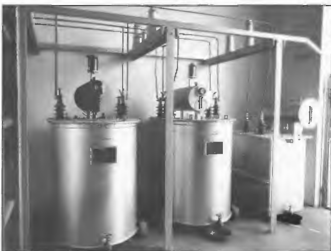
Oil filled vault equipment fitted with conservator tank and dehumidifier provided with STC 55 kW transmitters installed at NBS stations from 1958. The equipment was designed for either inside or outside mounting. This shows the SCL Adelaide system installed 1961.
