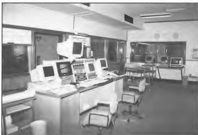
New control desk installed Radio Australia, Cox Peninsula 1993 as part of upgraded facilities to enable the station to operate with five 250 kW HF transmitters. Computer terminals for three Collins transmitters are at far end of room.
