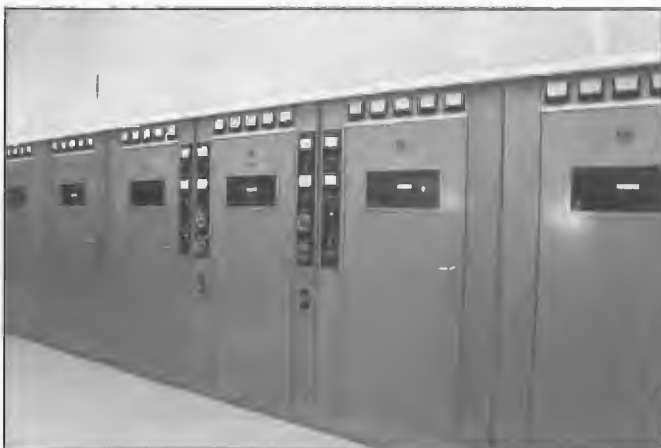
STC type 4-SU-61 50 kW HF transmitter at VLW Hamersley, Western Australia for ABC Inland service. It was installed in 1963 and was operational until 1994. It was the only transmitter of this type operational in Australia for broadcasting purposes. Band changing was achieved by using pneumatic rams remotely controlled by frequency selection switches in the driver unit.
