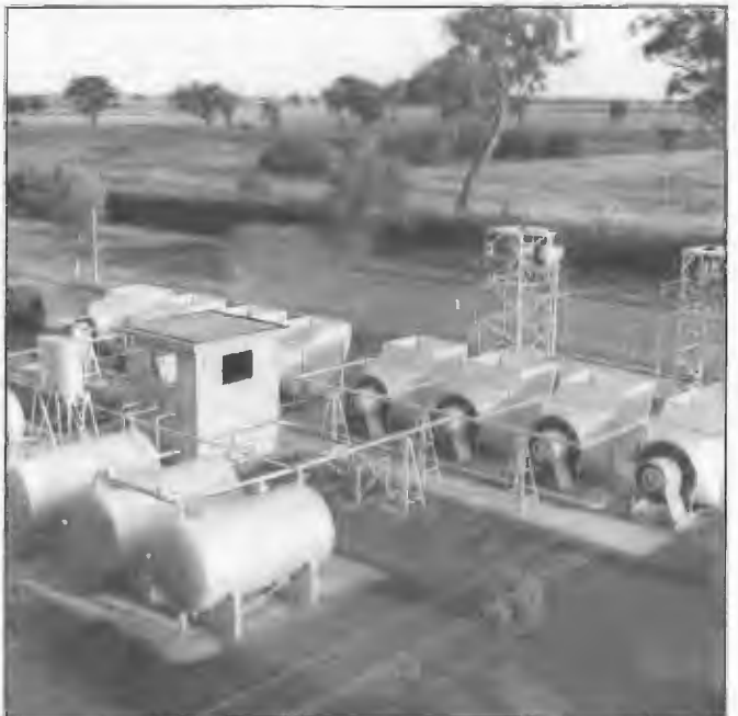
Outdoor water cooling systems for transmitters Radio Australia, Shepparton installed 1946. Water pumps were accommodated in the building while the air cooled radiators were installed outside.
