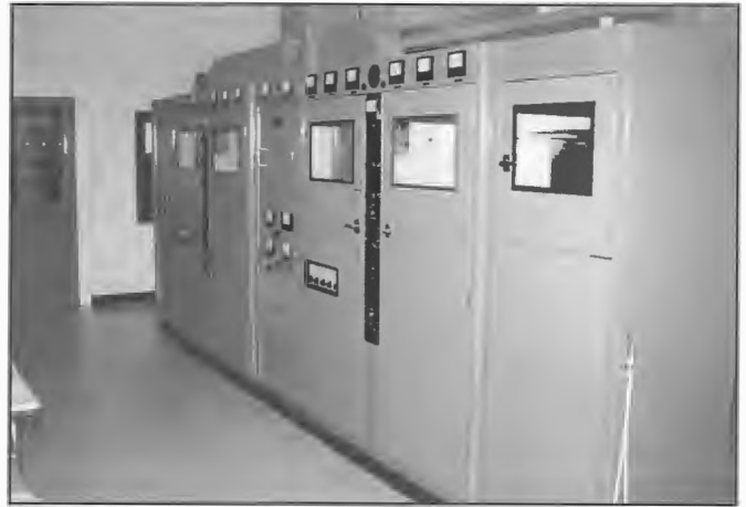
Twin STC 5 kW transmitters installed 5CK Crystal Brook 17 June 1966 operating in parallel mode. They fed into a sectionalised 190 m radiator via a six wire coaxial line.
