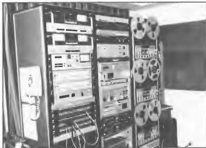
Station 3EON-FM Master control equipment. Transmissions commenced on 11 July 1980 with technical facilities being under control of Technical Director Neil McCrae. Facilities included three production control rooms, two on-air studios and a voice-over booth. The two larger control rooms were each fitted with a Sony fully automated console.
