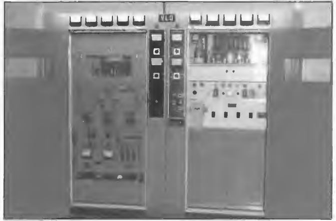
VLQ 10 kW transmitter STC type 4-SU-48B installed 1968 to replace A880A model. Final amplifier and modulator employed valve types 3X2500A3. Operational frequency was 9660 kHz. It was closed down during December 1993.
