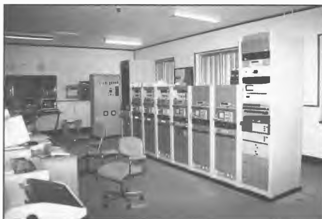
New program input equipment, monitoring and test racks installed at Radio Australia, Cox Peninsula 1993 as part of upgrading the station to accommodate two additional 250 kW transmitters. Aerial control panel and power supply mimic diagram in cubicle near end of racks.
