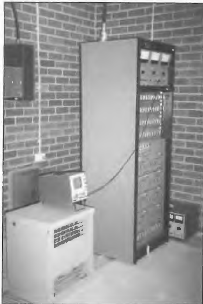
One of two Nautel 10 kW AMPFET 10 solid state transmitters installed at Viewbank, site of former Commercial station 3DB Melbourne. Callsign was later changed to 3TT and upon the owners of 3TT obtaining a licence to transmit on FM at another location, the AM facilities were transferred to the Commonwealth's National Transmission Agency. The two transmitters were used to provide an outlet for Parliamentary Broadcast Network station 3PB on 1026 kHz the former 3TT frequency and for an alternative standby transmitter for National station 3LO on 774 kHz for the Sydenham facility as from April 1993. The two transmitters had access to the aerial via a remotely controlled switching system.
