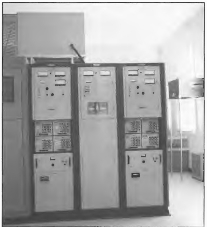
Two 5 kW ND5 AMPFET Nautel solid state transmitters operating in parallel at 5CK Crystal Brook March 1991. Each transmitter used four identical power sub-systems containing 3 FET power amplifier modules and its associated pulse duration modulator giving an output up to 5.6 kW per transmitter.
