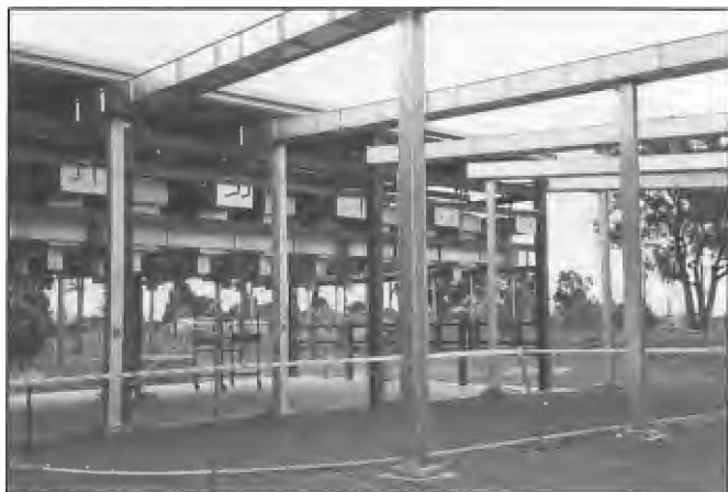
The 500 kW Marconi matrix switching system installed at Radio Australia, Shepparton 1991 to provide for seven transmitter inputs and 12 aerial outputs. The switch replaced an Australian designed and built system that had been in service for some 30 years. Project Engineers were Tech Chua and Mark Stevens with Kevin North and Doug Brodie being in charge of technical support groups.
