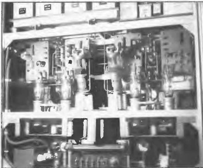
Final stage of 4QN Clevedon STC 6.25/7 kW transmitter commissioned in 1936. The stage employed a pair of 4220B water cooled valves with two on standby in spare sockets. The stage was a Class C amplifier with a pi type circuit terminated in a 600 ohm transmission line. The 12 kV EHT supply for the valves was supplied by a rectifier system employing three 4222A water cooled rectifiers.
