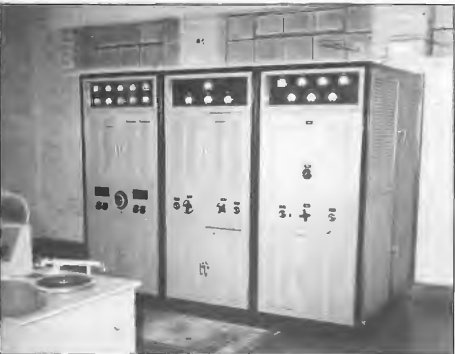
The 500 watt 3BA Ballarat transmitter manufactured by Transmission Equipment Pty Ltd and installed 1936 at Cardigan. It employed a 1 kW water cooled valve in the final stage and fed a 60 m high radiator. It replaced an old installation at another site. Chief Engineer (Transmitting Station) Warne Wilson.
