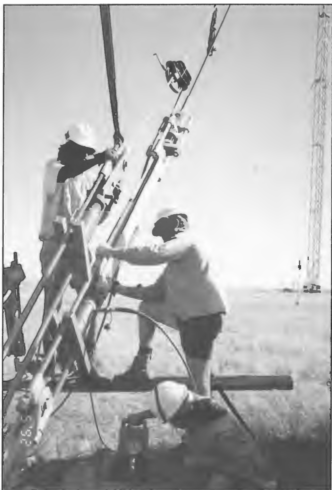
During 1992 Telecom staff undertook a program of works involving the replacement of guys at a number of major stations including 2BL/2RN Sydney, 3LO/3RN Melbourne, 5AN/5RM Adelaide, 5CK Crystal Brook, 5SY Streaky Bay and 6WA Wagin. Photograph shows replacement of one of the guys at 5SY Streaky Bay 137 m radiator. A temporary guy was installed to allow the working guy to be taken out of service and a new guy fitted. Project Co-ordinator Mike Dallimore.
