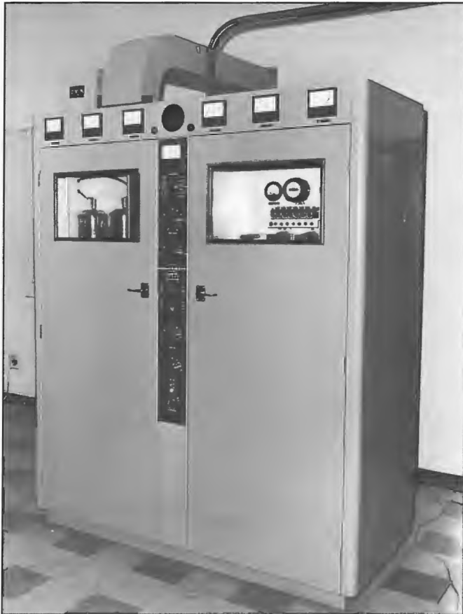
STC 2 kW transmitter installed at 5DN Adelaide 1964. The station transferred from the CML Building in the city to a site at Dry Creek in 1954 and installed new transmitting facilities and aerial system. Chief Engineer was George Barber.
