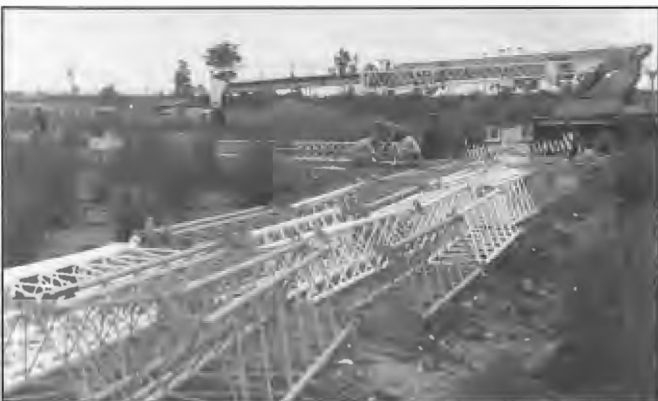
Assembly of 2HD Newcastle 134 m high lattice steel radiator prior to erection in 1983. The half wavelength structure was modified by the addition of a one eighth wavelength earth stub inside the lower portion of the mast to provide an electrically equivalent five wavelength anti-fading radiator. Chief Engineer at time of commissioning was David Suffell.
