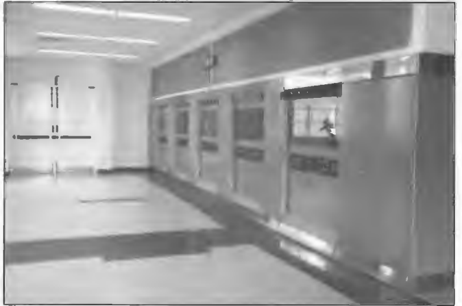
The STC 55 kW 3AR Melbourne transmitter was installed at Sydenham in 1962 sharing facilities with 3LO. The transmitter was replaced in 1991 by a Nautel ND25 25 kW solid state transmitter. The station now operates with callsign 3RN.
