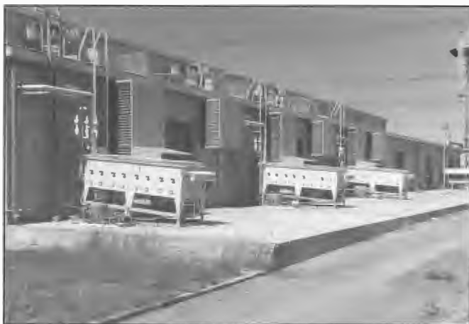
Steam condenser units provided for the vapour phase cooling system of three 250 kW Collins 821A transmitters at Radio Australia, Cox Peninsula. The station began transmissions in 1969 and was the first in Australia to employ vapour phase cooling of the high power stages. Project Engineer, Jack Ross.
