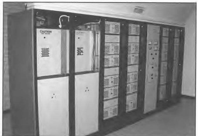
3WV Dooen 50 kW AMPFET50 Nautel solid state transmitter installed in 1988. It was the first solid state 50 kW transmitter to be commissioned in Australia. The power is obtained by using 48 identical 1.25 kW power systems combined into 5 kW groups. Twelve 5 kW blocks provide up to 60 kW output capability. Nautel transmitters are manufactured in Canada by Nautel Electronic Laboratories and distributed in Australia by JNS Electronic Industries.
