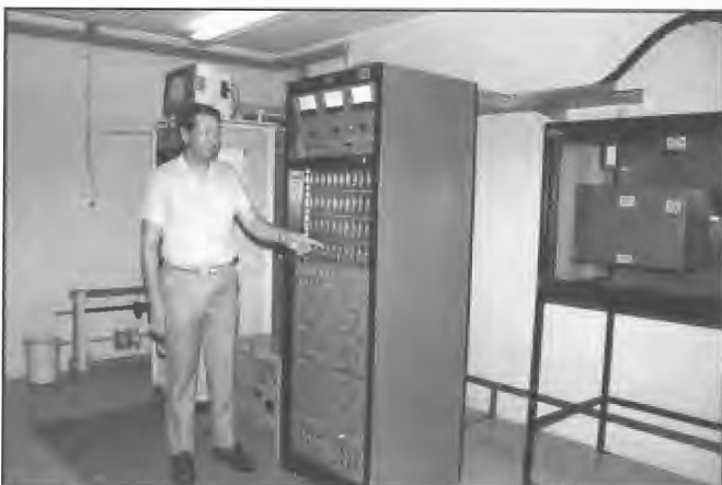
Nautel 10 kW AMPFET10 solid state transmitter commissioned at 4RK Rockhampton during 1988. Jeff Cirson, Officer-in-Charge at the unit. The transmitter was installed in a small building adjacent to the original building which had been erected in 1931.
