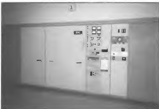
Brown Boveri 250 kW HF transmitter type SK53F3 installed at Radio Australia, Carnarvon 1976. Officer-in-Charge, Jack Clugston.
