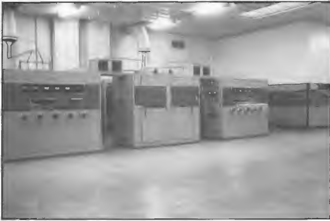
Modified STC/AWA 100 kW transmitters Radio Australia, Shepparton. Transmitters 3 and 4 in foreground and RCA 50 kW transmitter on right. The two original 100 kW transmitters were converted into four separate 100 kW units by using redundant and extra components during 1960s. Officer-in-Charge was Bill Davidson.
