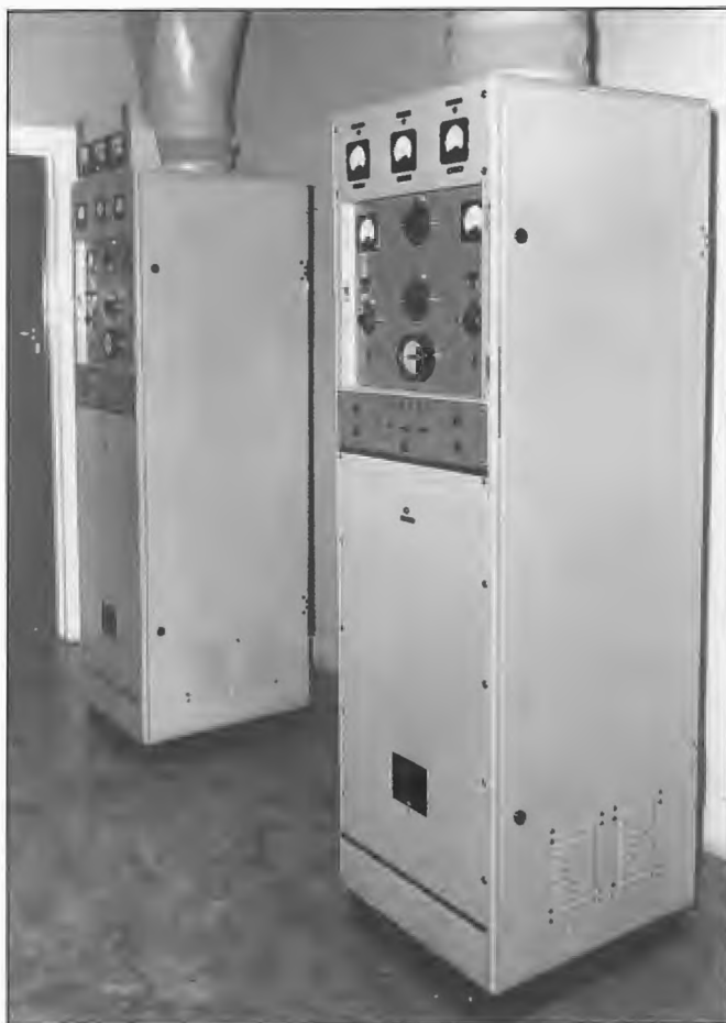
A pair of Philips 200 watt valve transmitters operating in main/standby mode at 5MG Mt Gambier. Commissioned on 26 September 1955, a similar installation had been provided at 5WM Woomera and operating on the same frequency. Installation Divisional Engineer was Murray Higgins and first Officer-in-Charge was Bill Legg. In 1974, the 5MG transmitters were replaced by a pair of STC 100 watt solid state transmitters operating in parallel.
