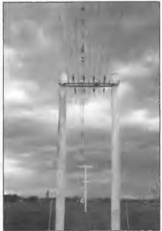
Nine conductor open wire transmission line in service at 10 kW NBS station 2KP Kempsey in 1994. It fed a 168 m anti-fading radiator. A similar line fed a standby radiator. This type of construction which utilised telephone line technology was employed at a number of stations in New South Wales and Queensland. The system comprised 4 active and 5 earthed wires and produced a characteristic impedance of approximately 100 ohms.
