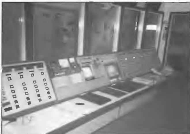
Station control desk Radio Australia, Carnarvon. The station was established in 1976 with a 100 kW Harris transmitter and a 250 kW Brown Boveri transmitter feeding four curtain aerials. Project Engineer, Terry Sellner.
