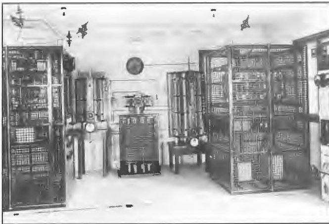
Part of an AWA 5000 watt transmitter installation at one station illustrating the method of interconnecting HT leads between units. Conductors were suspended from the ceiling with strain type porcelain insulators fitted with corona rings. Units (L to R) Magnifying unit, tuning inductors and capacitor, and HT rectifying unit. The wall lead-through insulators for aerial and counterpoise feeds are in the centre. The counterpoise feed point is partially obscured by components. AWA Construction Engineer D Campbell.
