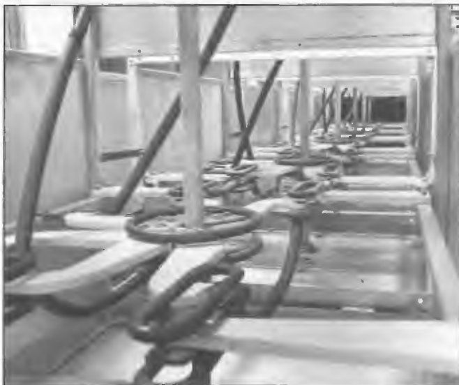
Ceramic switching arms and phosphor bronze contacts of Brown Boveri transmission line matrix switch Radio Australia, Cox Peninsula 1969. The switches were remotely controlled from the station control room.
