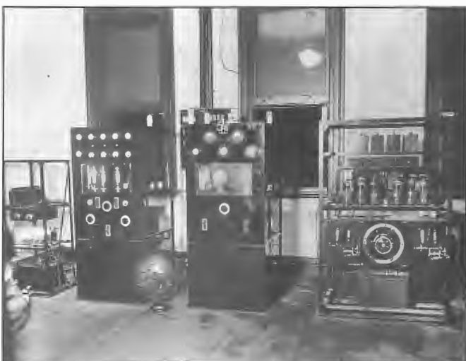
Original 5AD Adelaide transmitter constructed by station staff under Harry Kauper and put to air in 1930. Originally, the final stage employed two air cooled valves in parallel to provide 300 watts to the aerial but were replaced by an STC 4228 water cooled type. Further changes took place over the years until it was replaced by an STC 2.5 kW model in 1954 at Cavan.
