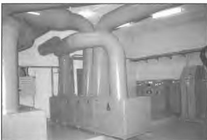
Filtered air ventilation systems with 250 kW Thomson—CSF TRE 2326 transmitter installed Radio Australia, Cox Peninsula 1993–94. A high pressure system provided air to the RF stage while a low pressure system catered for the Modulator stage. Equipment mounted to the right comprised 11 kV switchgear and 11 kV/400 V step-down transformer. Contractor's installation and commissioning staff comprised Marc Moreau, Guy Pellett and Didier Thomas.
