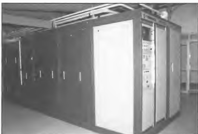
Thomson-CSF TRE 2326 HF 250 kW transmitter commissioned Radio Australia, Cox Peninsula 1994. Two identical transmitters were placed in operation bringing the total 250 kW transmitters at the station to five. A video colour display module incorporated in the transmitter control panel indicated the transmitter status. In the event of a fault, plain language messages were displayed in conjunction with faults to assist in fault resolution. Project Engineer, Graham Baker.
