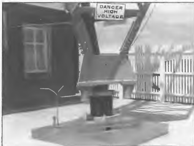
Base insulators at the base of the 5CL/5AN 172 m dual frequency radiator 1961. The insulators are unusual in that they comprise four porcelain cylinders filled with oil. Similar unit were installed at 5CK the following year. The insulators were imported from USA by the contractor Electric Power Transmission. Divisional Engineer, Jack Ross. Line Inspector, Don Beames.
