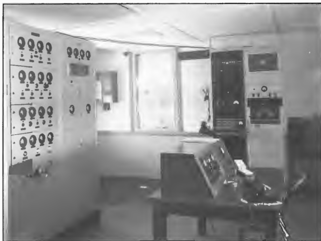
STC 1 kW 6WN transmitter installed at Canning Bridge 6 km south of Perth. The transmitter had operated at 500 watts from the Perth GPO since 1938 but with the outbreak of hostilities with Japan in 1941, the transmitter was moved to a bushland site at Mt Lawley and later relocated to Canning Bridge in 1946.
