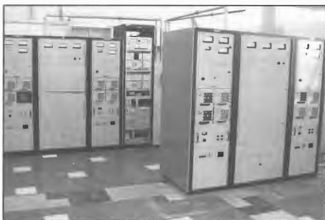
Nautel ND5 solid state transmitters installed at NBS station Dalwallinu during late 1994. Two ND5 units are combined to produce 10 kW to line for each service. The front unit caters for a new Radio National service 6RN while the rear unit is associated with Regional service 6DL. Station 6DL has been operational since 22 November 1963.
