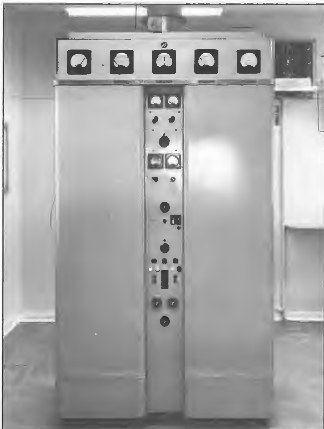
AWA 200 watt valve transmitter 5LN Port Lincoln commissioned 14 November 1950. Identical main and standby units were provided. First Officer-in-Charge was Jack Martin. In 1974, the valve transmitters were replaced by a pair of STC 100 watt solid state units operating in parallel mode. In 1998, a new 200 watt transmitter replaced the STC units.
