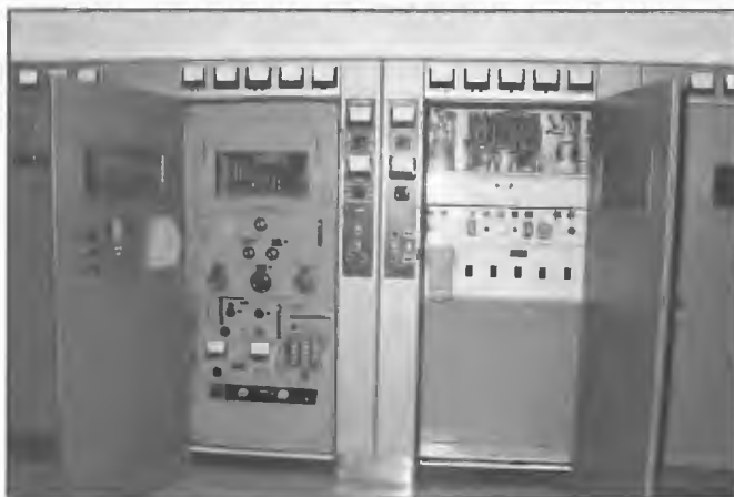
Front view of STC 10 kW transmitter type 4-SU-48B installed in 1963 and operational at Hamersley until 1994. Two were in service covering the 6 and 9 MHz bands. The design was employed as the driver unit for the 50 kW transmitter also in service at the station.
