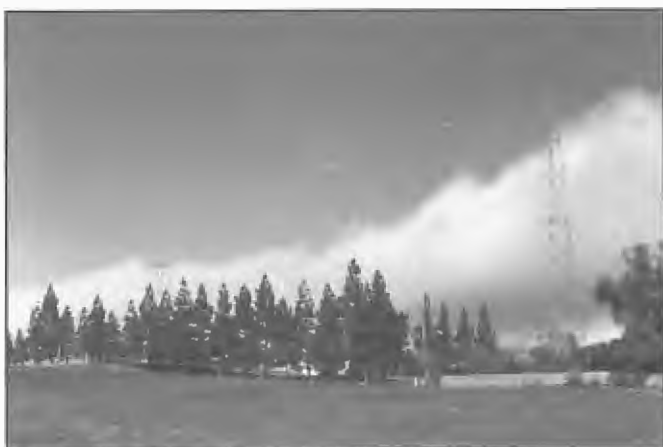
Multiple tuned or Alexanderson aerial system installed at 5CK Crystal Brook in 1932. Similar systems were installed at 2CO Corowa and 6WF Perth and were still operational 60 years later, mainly as standby units. The multiple tuned aerial was developed by Ernst Alexanderson a prolific USA inventor with 290 Patents to his credit.
