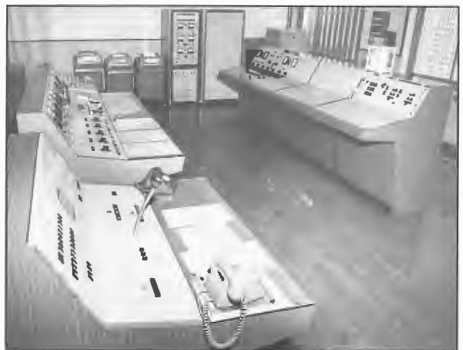
Control room Radio Australia, Cox Peninsula 1969. Facilities included communications, program input, frequency selection, aerial switching, transmitter digital control, emergency power and gate surveillance equipment. Design Engineer, John Robertson.
