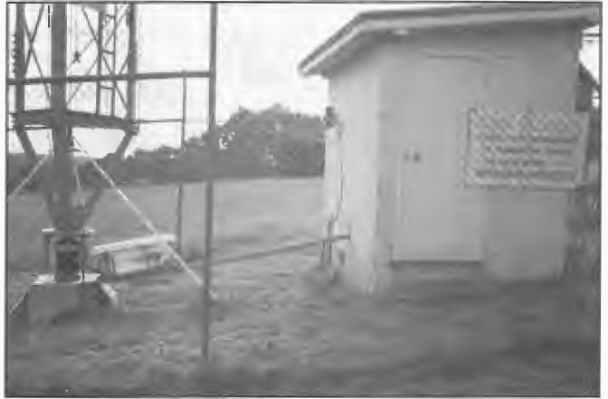
Base of the 134 m high lattice steel radiator at 3RPH Melbourne showing the base insulator, grounding system and lightning arrester. The system was originally commissioned in March 1956 for Commercial station 3KZ Melbourne when approval was given for Melbourne based stations to be transferred to Heidelberg-Lower Plenty area and for transmitter powers to be increased to 5 kW. Transmission line is a six conductor open wire type. The facility was transferred to the Print Handicapped group with callsign 3RPH when the owners of 3KZ acquired a licence to operate in the FM band from 1 January 1990.
