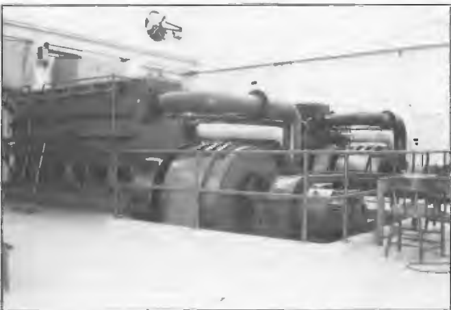
Emergency power plant Radio Australia, Shepparton installed during the 1940s and comprising two Crossley 800 HP diesel engines each coupled to a 400 kW Brush alternator. Equipment operated as a synchronous pair and remained operational until 1993 when it was taken out of service. Staff who worked on the engine generator equipment at various times included Dick Cox, Brian Bingham, Steve Nankivell and Keith Dahlberg.
