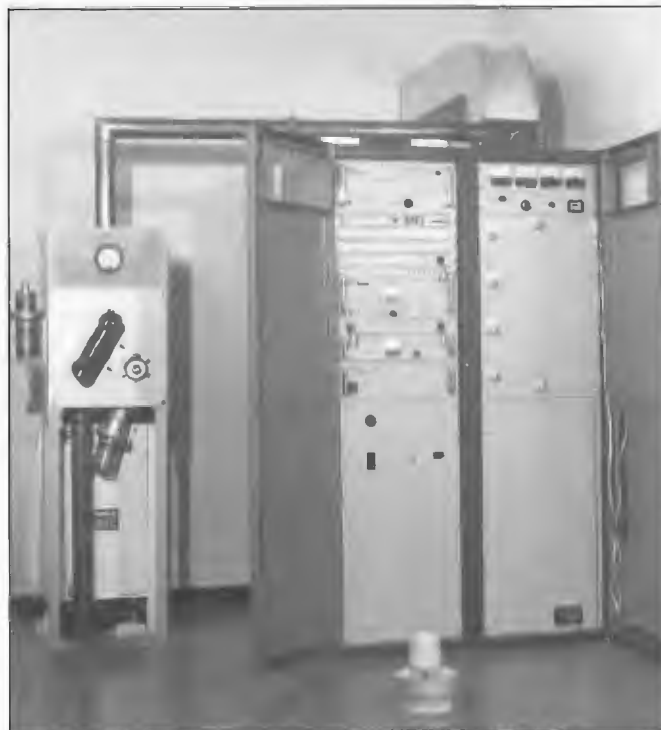
NEC 10 kW FM transmitter installed at Mt Gambier 1981. The output valve employed is displayed in front of the transmitter. This is typical of many FM transmitters installed throughout Australia for the ABC FM Stereo service which began in 1986. Officer-in-Charge, Rawdon (Ron) Mitchell.
