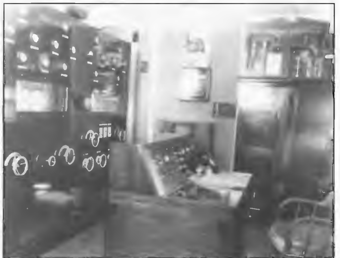
STC 2 kW water cooled transmitter 4RK Rockhampton and control desk circa 1936. The desk included a General Radio Modulation Monitor type 731A. The floor mounted monitoring loudspeaker replaced a WE 560-AW table model provided in 1931 when the station was commissioned. Officer-in-Charge 1931-36, Harry Conway.
