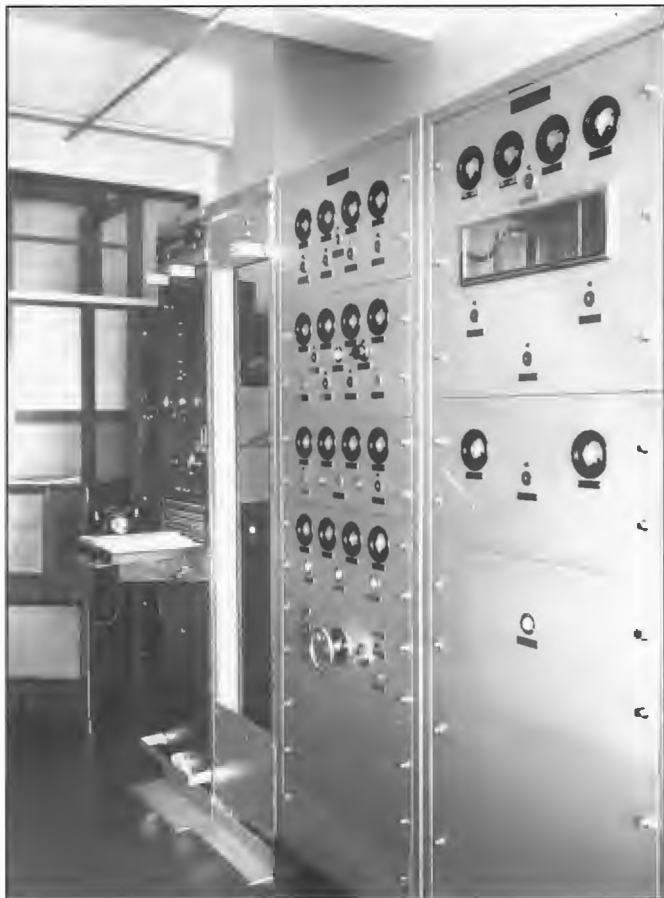
Original STC transmitter installed on 6th Floor, Perth GPO when 6WN was commissioned on 12 October 1938 on frequency 790 kHz. The final linear amplifier stage comprised a pair of 4279A valves in push-pull and produced 500 watts output. The design by STC was intended to cater for a range of transmitter powers in the range 50 to 2000 watts to meet the needs of Commercial and National broadcasters in the 1930s.
