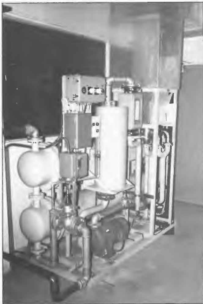
Water cooled 500 kW dummy load installed at Radio Australia, Carnarvon 1976 for testing 100, 250, and 300 kW transmitters. The station ceased operation in 1996. Officer-in-Charge when station closed, Les Fancote.
