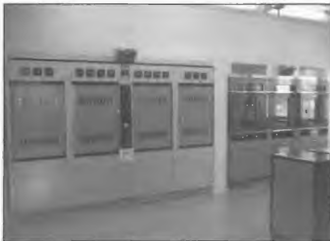
NBS transmitting centre Newcastle. Left, 2NC 10 kW AWA BTM10 transmitter and on right, 2NA 10 kW Collins 21E/M transmitter. The first 2NC transmitter was commissioned on 19 December 1930 followed by 2NA in 1943. The two 10 kW transmitters were installed in 1959.
