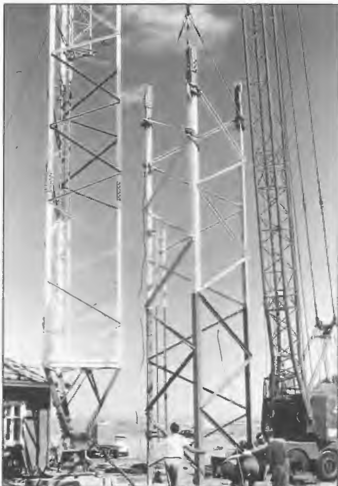
The erection of lattice steel masts for broadcasting purposes, calls for a high level of skill and considerable field experience. During the erection of the lower sections of the mast a crane is often used. When the 172 m 5CL/5AN radiator was erected in 1961 a crane assisted in the erection of the bottom sections up to about the first permanent guy point. The structure was placed on wooden blocks until the first level guys had been installed. Hydraulic jacks lifted the structure to allow the base insulator to be put in place. Contractor Electric Power Transmission, Sydney.
