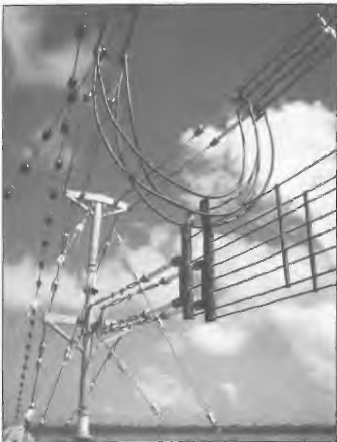
Steel support and terminating poles create a problem when located in areas of high field intensity and break-up insulators are frequently employed for poles and stay ropes. The photograph shows a sectionalised pole located at the feed point of a dual plane log periodic aerial fed by 250 kW transmitter at Radio Australia, Cox Peninsula 1969.
