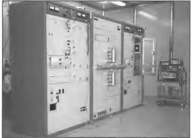
Typical dual 10 kW NEC FM transmitters undergoing tests in the manufacturers screened room 1990. NEC was the largest supplier of FM transmitters in Australia and assembled 10 kW and 20 kW transmitters at its Mulgrave Broadcast Engineering Centre near Melbourne from imported sub-assemblies and locally sourced items. Roger Greenwood was Manager NEC Broadcast Systems.
