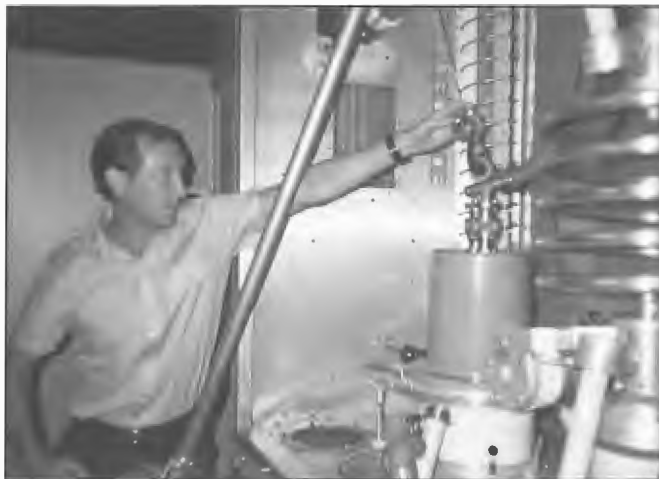
The replacement of bulky and heavy transmitting valves has been a problem with maintenance staff for many years. However, today only high power HF transmitters in Australia use large valves for radio broadcasting purposes. All stations were equipped with lifting facilities to enable replacement of a valve by a single operator. Photograph shows Phil Leaney operating a lifting device for replacement of a Thomson TH573 valve in a 300 kW Thomson transmitter at Radio Australia, Carnarvon before closure of the station in 1996.
