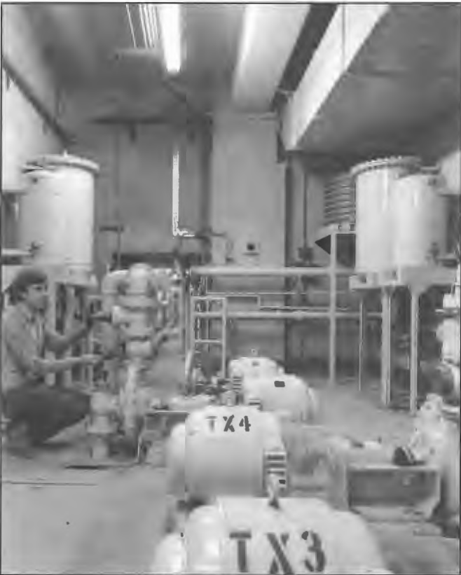
Water pumps and associated equipment for removal of heat from the anodes of the high power valves Radio Australia, Shepparton. Air cooling ducts are also visible. Part of the original 1946 installation.
