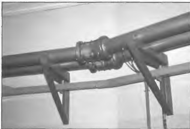
Rigid coaxial lines installed at 5CL/5AN Pimpala 1961 to allow connection between transmitter output circuit and the outside unbalanced 200 ohm transmission line. The coaxial lines were maintained under pressure with dry air. Manufactured in PMG's Department Adelaide Workshops. Installation Supervisors, Don Beames and Frank Henschke.
