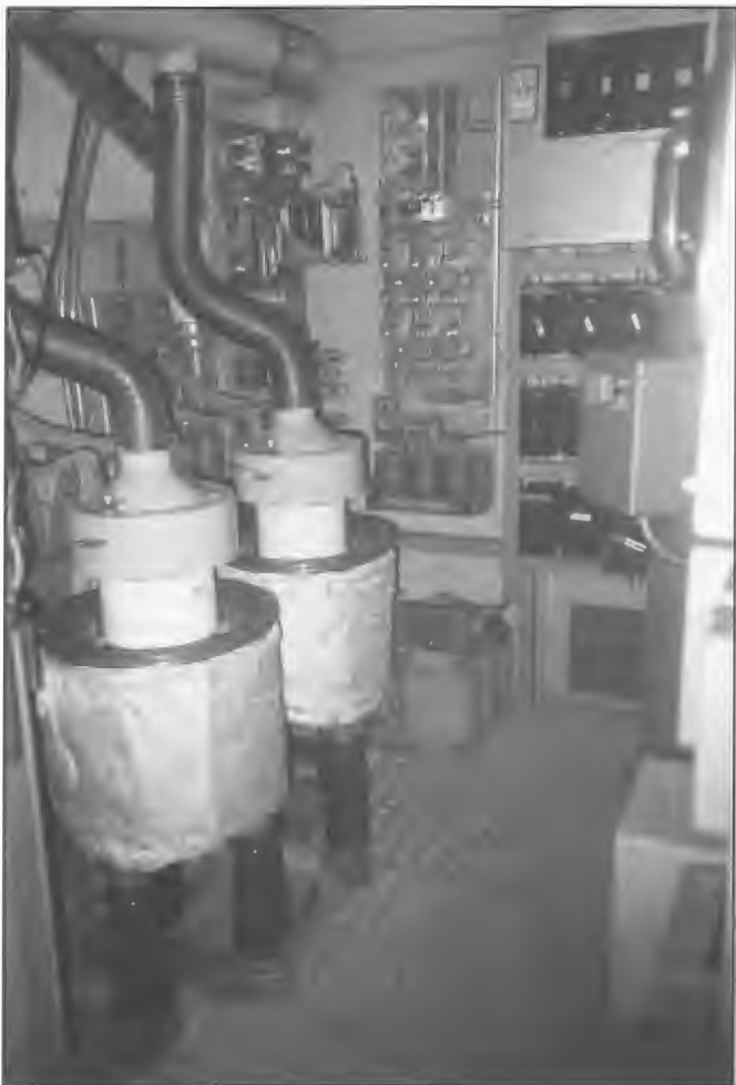
Valve type CQS50 ceramic tetrodes in push-pull in the modulator stage of the 250 kW Brown Boveri transmitter at Radio Australia, Carnarvon. The modulator employed conventional high level modulation with modulation transformer and choke. Transmissions commenced 20 December 1975. Murray Little and Trevor Chapman were members of the installation team.
