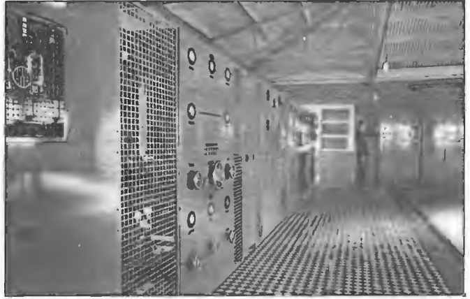
Transmitter constructed by Amalgamated Wireless (A/Asia) Ltd and installed at the AWA Radio Centre Pennant Hills for Commercial station 2SM circa 1935. The transmitter was maintained by AWA technical staff for the owners of 2SM, Catholic Broadcasting Company. The transmitter with 1 kW output employed series modulation in which the modulating valve was connected in series with the anode potential supply of the valves of the high frequency amplifier of the transmitter.
