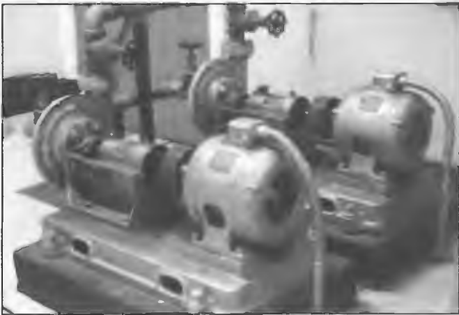
Duplicate water pumping system installed at VLQ Bald Hills 1943 as part of cooling facility for 10 kW STC transmitter type A880A which employed SS1971 type valves and later 3Q213E type. The 2-3/4 HP motor circulated distilled water to the valve anodes at rate of 6 gallons per minute. Divisional Engineer in charge of installation was Vern Kenna.
