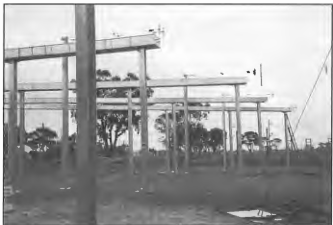
With the commissioning of five broadband aerial systems and associated transmission lines in late 1993 for Radio Australia, Shepparton, the transmission lines were extended as enclosed lines for some distance from the matrix switch before changing to four wire open wire types to minimise cross coupling effects between adjacent lines.
