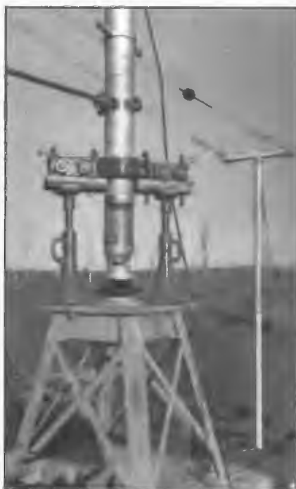
Jacking arrangement to lift the 4AT radiator to enable base insulator to be placed in position. The radiator put into service in 1961 replaced the original which had been in service since 1939.
