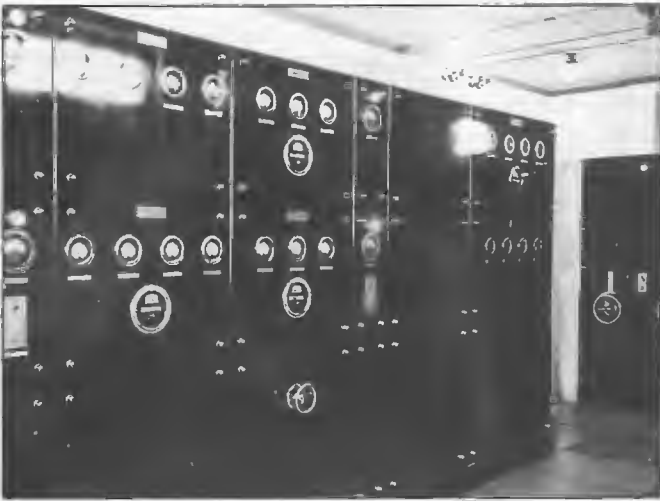
Front view of 3GI Sale transmitter. Similar units were provided for 7NT, 2NR, 4QN and 6GF in the mid 1930s. The final amplifier employed a pair of 4220B water cooled valves. With the exception of the final stage, power for all filament and anodes was provided using copper oxide rectifiers. The EHT was provided by three water cooled 4222A diode valves. Divisional Engineer Harold Robertson.
