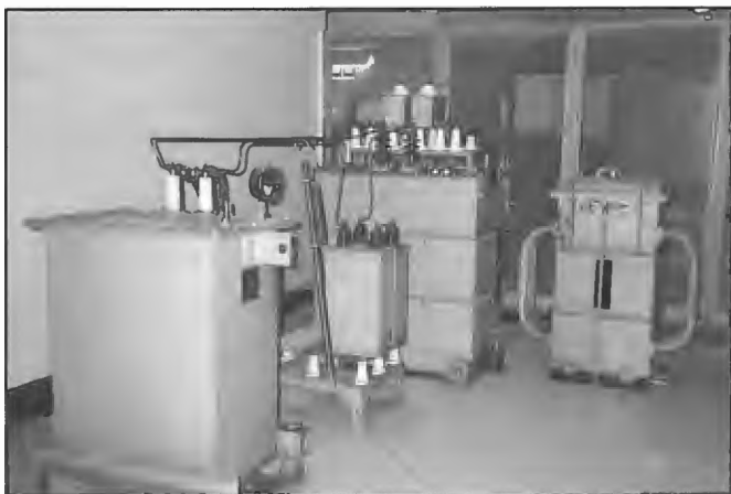
Heavy components associated with modulation circuitry of 10 kW transmitter STC 4-SU-11A operated during 1994 as 4PB Brisbane. Large components were a characteristic of designs employing high level modulation. The transmitter located at NBS station Bald Hills near Brisbane was manufactured in 1948.
