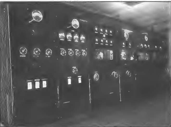
5CK Crystal Brook 6.75 kW STC transmitter commissioned 15 March 1932. An identical unit was installed at 2CO Corowa. Installation engineers were Frank O'Grady and Laurie Billan. The transmitter remained in service for 20 years.
