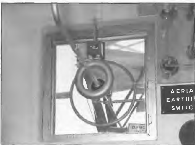
One of a number of RF current transformers installed at 5CL/5AN Pimpala 1961 designed for 50 kW application. The transformer was developed by Phil Humphries, STC Engineer Sydney based on an STC England model provided for the BBC. The Pimpala station was the first station in Australia to be fitted with this type of current transformer. Major advantages were that it could handle high RF currents and voltages and did not involve a break in a conductor for insertion of a meter. Divisional Engineer, Jack Ross.
