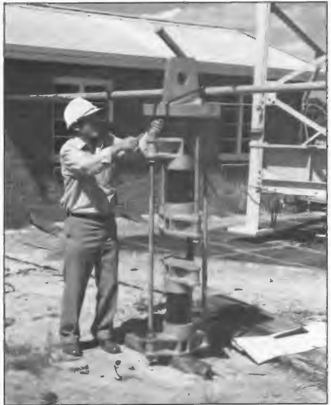
Guy insulators for 180 m 6WF/6WN radiator guy system being prepared for installation by Project Engineer, Alan McCarthy 1986. The mast was erected in 1953 and the design of the original insulator mount was such that some operational problems had occurred due to arc-over. Senior Lines Officer, Stan Randall controlled the workforce, Senior Draftsman, Ian Gibbs checked mast alignment and Structural Engineer, Bruce Cook provided specialist advice.
