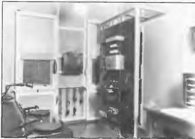
Speech input equipment racks and emergency studio 4RK Rockhampton circa 1936. Pick-ups are Western Electric 4A oil damped gramophone reproducer units employing steel needles. The microphone is a type 633. The station was commissioned in 1931 but equipment shown was provided later.
