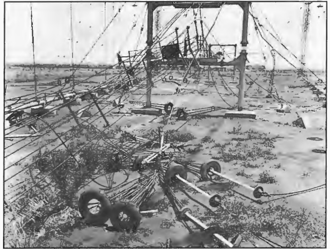
Damage to the dual plane log periodic transmitting aerials at Radio Australia, Cox Peninsula as a result of Cyclone Tracy 1974. The cyclone struck the station shortly after midnight on Christmas Eve December 1974 with winds estimated at 200 kilometres per hour. All five aerial systems and associated transmission lines were badly damaged.
