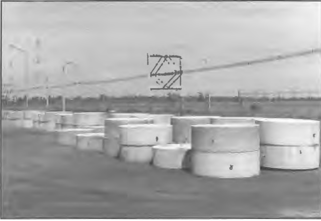
Concrete counterweights assembled on site prior to attachment to catenaries supporting the Radio Australia, Cox Peninsula aerial systems 1984. Seven arrays were supported by lattice steel guyed masts 47, 67 and 97 m high. Construction staff included Volka Lange, Graham Hooper and Jim Finch.
