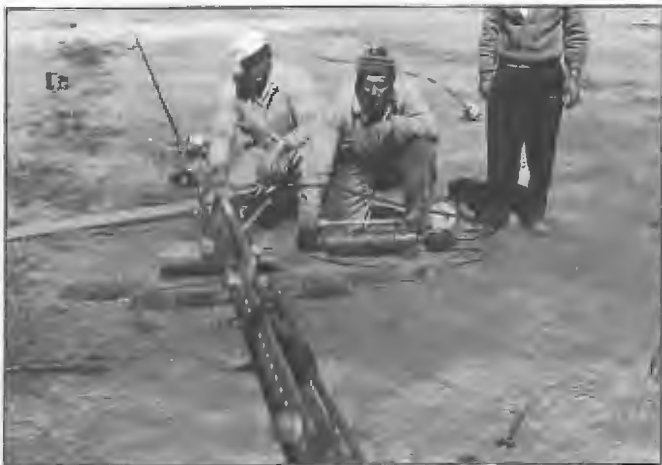
On site test bed facility employed for pretensioning guy ropes installed with 5CL/5AN Pimpala 172 m radiator May 1961 and 5CK Crystal Brook 190 m radiator February 1962. Work was carried out by Electric Power Transmission, Sydney. The pretensioning operation checked all elements including insulators and eliminated non elastic stretch which would occur over a period of time in service requiring subsequent guy tension adjustment.
