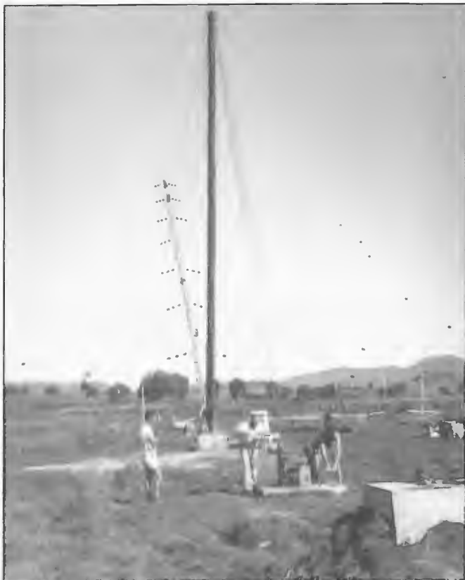
Erection of 61 m high 150 mm diameter pipe radiator 1961 for 4AT using falling jury method. The jury pole was 22 m high. A hand operated winch was used to pull the radiator to the vertical position. Electrical Design, Ron Tolmie; Structural Design, Clyde Manuel; and erection team under control of Duncan Russell-Hall.
