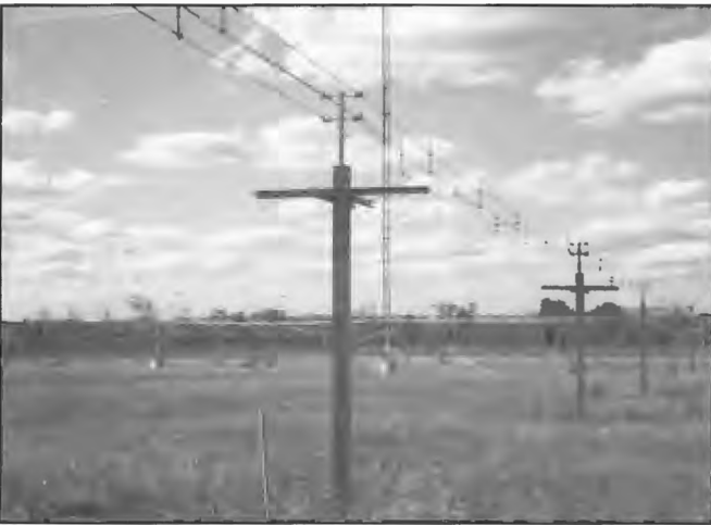
Four wire 300 ohm balanced transmission line using alumoweld supported by steel poles provided at NBS high frequency broadcasting stations at Alice Springs, Tennant Creek and Katherine 1986. Senior Engineer, Bruce McGowan.
