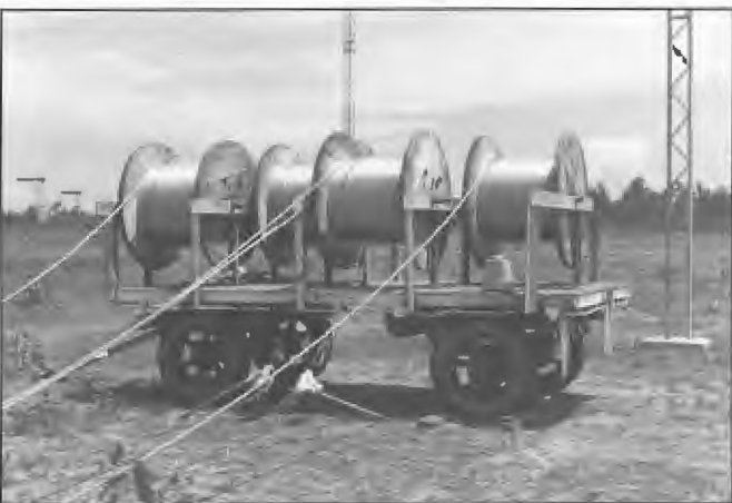
Drums of alumoweld wire used during assembly of seven curtain aerias for Radio Australia, Cox Peninsula 1984. Alumoweld has an inner steel conductor surrounded by aluminium giving the conductor high strength, good conductivity, high resistance to corrosion and light weight compared with copper. Station Engineering Manager, Graham Shaw.
