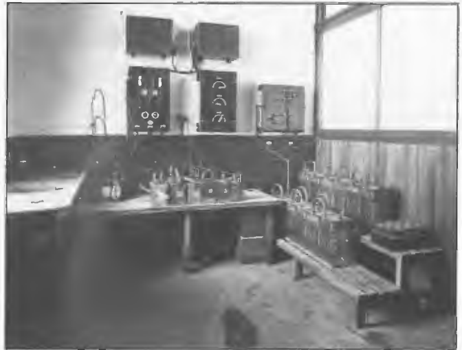
The battery room at 3LO Melbourne 1924. At the time all power requirements of valves was provided by A,B and C type batteries. The A batteries were usually accumulator types. It was not until 1935 that suitable valves became available for operation of filaments using AC.
