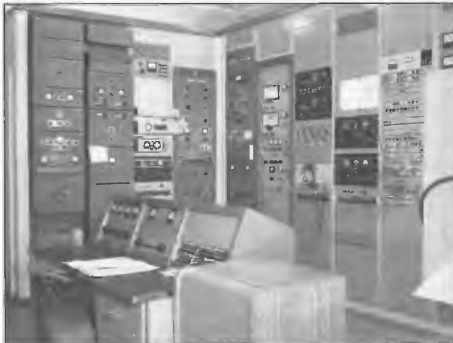
Receivers and aerial patching facilities at High Park Receiving station 1959. In the period between its establishment in 1959 and closure in 1986, the station played an important role in reception of programs for rebroadcasting by the ABC. At time of closure, station Officer-in-Charge was Peter Dainton.
