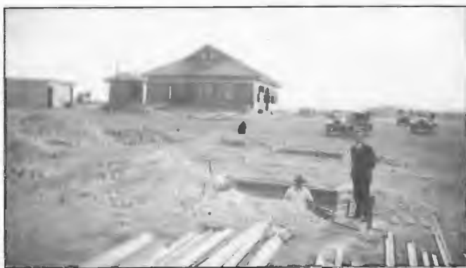
Installation progress at 5CK Crystal Brook 1931. Workman of tower erector Messrs Gibb and Miller, Port Adelaide preparing foundations watched by Engineer Laurie Billin. Material for the two 56 m high lattice steel structures was supplied by Johns and Waygood Melbourne.
