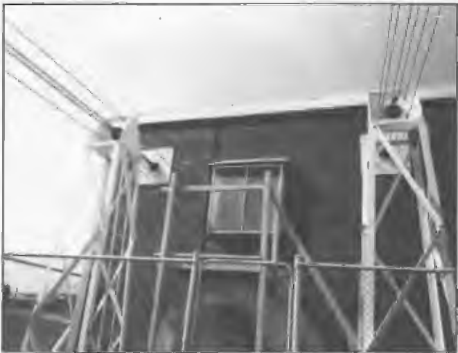
Terminating towers and universal terminating and lead-in type porcelain insulators for 10 kW standby transmitters 5AN/5CL Pimpala 1960. The double bowl insulators were held together by a stud so that the two bowls were in compression when installed. The assembly was much stronger than a single bowl which was usually attached by several brackets or bolts. Design Engineer, Bill Gold.
