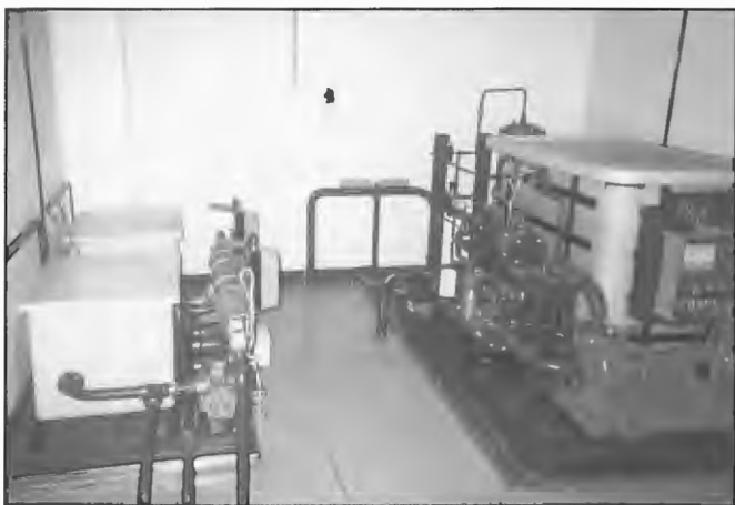
Water cooling equipment for valves and capacitors with the 300 kW Thomson-CSE TRE2320 transmitter installed at Radio Australia, Carnarvon in April 1984. Prior to closure of the station in mid 1996, the transmitter was the most powerful in the Radio Australia service. Officer-in-Charge at close down, Les Fancote.
