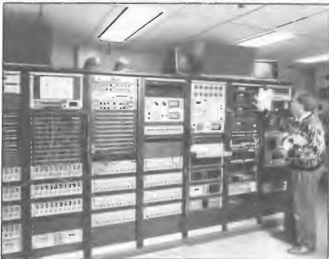
Tom Rowan, Transmission Supervisor in Master control room of the ABC Radio Australia studios Burwood East, Melbourne 1988. At the time, 16 Aussat lines plus terrestrial lines came into the Master control room and 20 lines were available to serve Radio Australia transmitters at Shepparton, Carnarvon, Cox Peninsula and Brandon.
