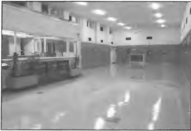
Transmitter Hall, Lyndhurst transmitting station 1986. Control room is on left. The station was established in 1928. In the late 1960s eight new STC 10 kW transmitters were installed to cater for the many commitments provided from the station. Its functions gradually declined and the station was closed down on 12 June 1987. Officer-in-Charge at closedown was Max Fowler.
