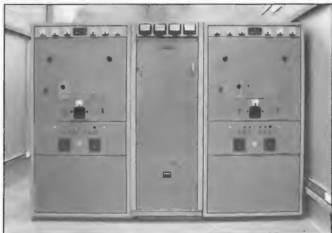
Parallel 1 kW STC transmitters with combiner installed at 3MT Omeo on 18 April 1976. The transmitter employed power amplifier valve types 5/500A with HT being supplied by a silicon rectifier system. Aerial system was a 108 m directional type with two masts.
