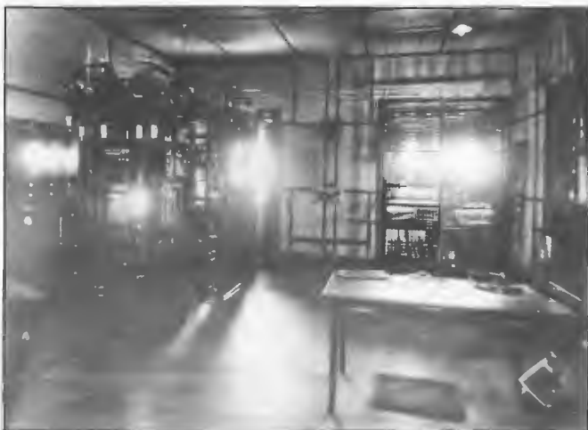
Original AWA 5 kW transmitter installed at 5CL Adelaide 1925. The transmitter was modified by Chief Engineer Harry Kauper in 1927 and equipped with WE4220B water cooled valves to replace the air cooled types in the high power stage. The transmitter was replaced in 1936.
