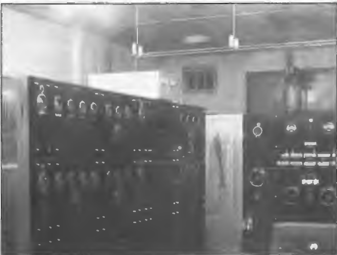
The original 4QN STC 6.25/7 kW transmitter installed at Clevedon November 1936. Installation Foreman was Reg Baker and first station Officer-in-Charge was Les MacDonald. The transmitter was destroyed by fire on 26 May 1951 when Officer-in-Charge was Geoff Beetham.
