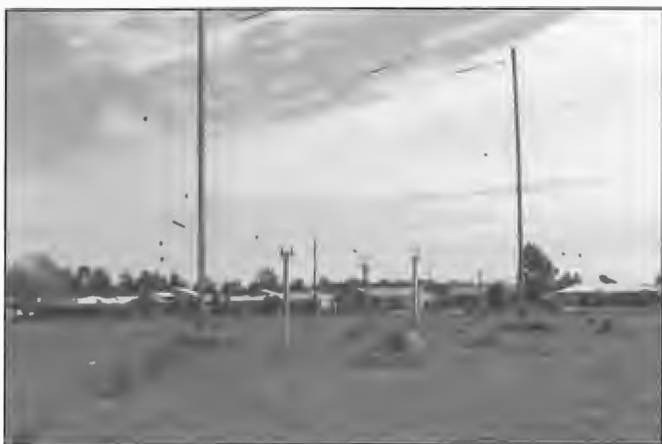
Part of VLQ aerial system installed at Bald Hills 1943 using dipole and reflector format. Support structures were sawn Oregon masts. Transmission line was 600 ohm two wire type. The service which transmitted ABC programs was closed down in December 1993. Vern Kenna was in charge of installation.
