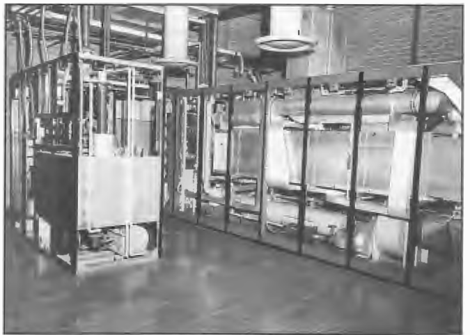
One of the 250 kW Collins 821A transmitters at Radio Australia, Cox Peninsula during installation stage 1969. Modulator stage on left. On right is power amplifier stage with cavity tank circuit, balanced to unbalanced transformer and band pass filter. The employment of a cavity for the tank circuit was a radical departure from the usual coil/capacitor arrangement.
