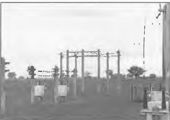
Wooden poles were used for many years for support of aerial systems at receiving stations and transmission lines at transmitting stations. The disadvantage of such practice outweighed the advantages and today are not employed. At Radio Australia, Shepparton wooden poles served the purpose for about 50 years from the 1940s before being replaced by steel poles when new aerial systems were provided in 1993.
