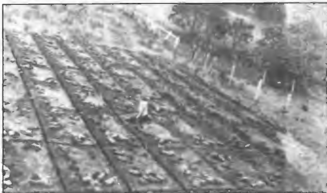
In the 1920s and early 1930s earth mats associated with aerial systems were laid as a grid, fishbone, a combination of these or as in the case of 7ZL, a rectangular grid with two semi circular radial systems. These systems were laid in trenches dug by hand. The 7ZL mat was laid in December 1926. Construction Engineer Donald Macdonald.
