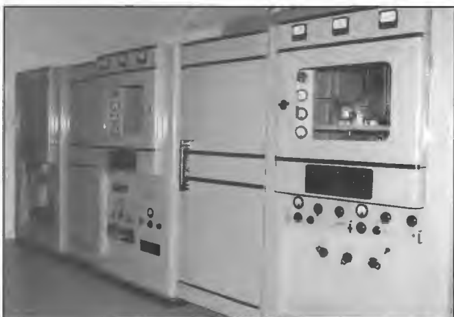
STC 10 kW transmitter type 4-SU-11A commissioned at 4RK Rockhampton 15 September 1954. It was painted Corio Sand colour, a colour scheme STC also used with some 2 kW models. The 10 kW transmitter employed high level modulation with the modulator and final power amplifier employing 3J221E triode valves. The EHT supply of 10 kV was provided by six 4078Z HCMV valves. The transmitter remained in service until 1988. Installation staff, Gordon Gilbert, Ian Byrnes and Col Williams.
