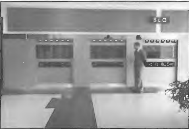
STC 55 kW transmitter installed at 3LO Melbourne 1962. Officer-in-Charge, Russell Rolls standing near the transmitter. It shared the 214 m radiator with 3AR. The site located at Sydenham was established in 1938 to accommodate 3LO and 3AR on a common site. The STC transmitter was replaced in 1991 by a twin 25 kW Nautel ND25 solid state installation.
