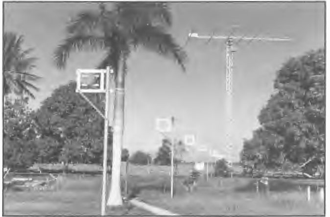
Rotatable aerial installed at Radio Australia, Brandon 1989. The system had previously been in service at Lyndhurst. The support tower is 32 m high. The aerial has an input impedance of 120 ohms and a tapered transmission line is used to match the transmitter to the aerial. The rotatable log periodic aerial was manufactured in the 1960s by Standard Telephones and Cables Pty Ltd, Sydney. It covered the frequency range 4 to 30 MHz. Boom and elements were made from extruded sections of aluminium-magnesium-silicon alloy.
