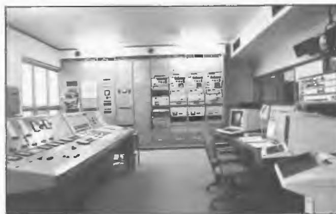
Control room, Radio Australia, Cox Peninsula after recommissioning in 1984 following extensive damage by Cyclone Tracy in 1974. Program input equipment racks in background, aerial and power control desk to the left and main control desk to the right. Officer-in-Charge was Ross Kearney.
