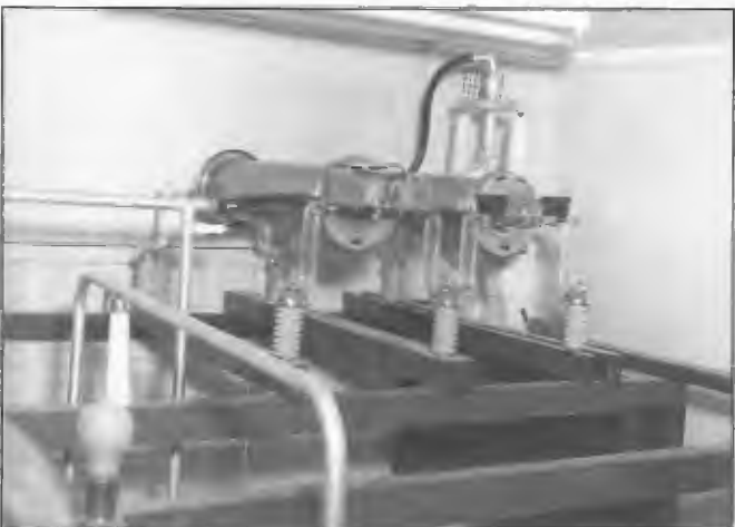
Twin RF chokes provided in mast lighting AC feed to 172 m 5AN/5CL Pimpala radiator 1961. The gradient wound chokes were designed by Bill Gold and installed by Frank Henschke. The chokes prevented RF leakage back to the station via the AC mains through capacitance leakage across the transformer. The wood used in the coupling hut structures was jarrah recovered from an old building erected alongside the Adelaide Telephone Exchange Building in the 1920s and dismantled in 1960. All fixings timber-to-timber were by wooden pegs.
