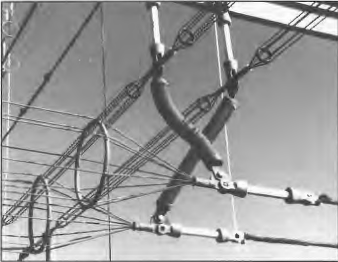
At Radio Australia stations where open wire transmission lines are employed, it is necessary to change direction of many lines and care needs to be taken in the layout design and construction to ensure the change takes place without introducing a change in the characteristic impedance of the line. The photograph shows the technique employed at Carnarvon installed 1975 and designed by Brown Boveri Co.
