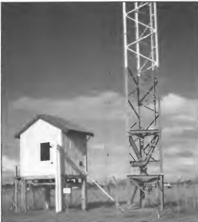
Typical base insulator mounting arrangement at a site subject to flooding. The 2KP Kempsey sectionalised radiator base insulator and the aerial coupling unit are mounted 2.5 m above ground level. The 168 m sectionalised radiator was erected in 1954 and in 1965 was fed by a pair of STC type 4S55B 5 kW transmitters in parallel. The mast is located on a flood plain alongside the Macleay River and flooding of the site is a frequent occurrence.
