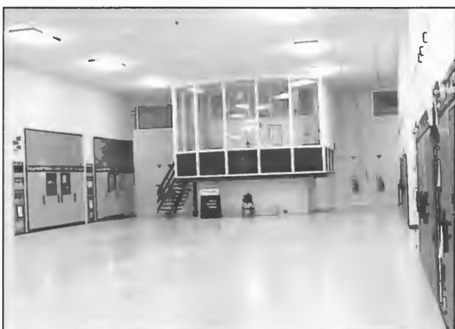
Radio Australia, Shepparton transmitter hall 1994. (Centre) Program Control Room; (Left) Transmitters 5 and 6, Harris SW100, 100 kW transmitters installed 1978; (Right) Transmitters 1, 2, 3 and 4 Harris SW100A, 100 kW transmitters installed 1983. Officer-in-Charge, Bruce Wilson.
