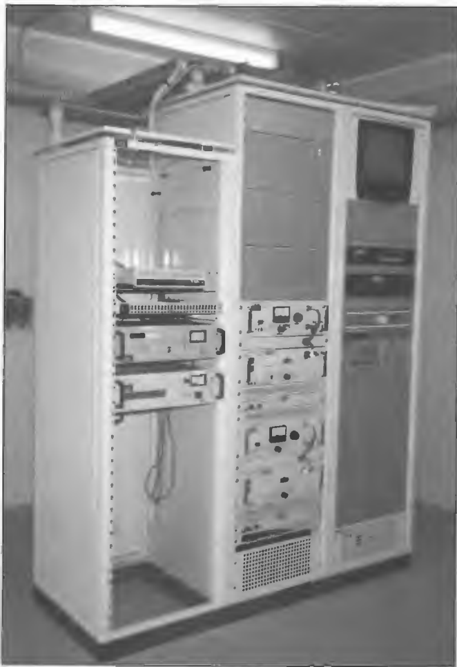
CTE FM transmitter installed at Gladstone in 1993 by Telecom Broadcasting for TAB as part of its Racing Radio Network. Programs are sourced from 4TAB, the TAB's station in Brisbane and relayed to other stations throughout Queensland via satellite. The Gladstone station was one of 16 installed during 1993.
