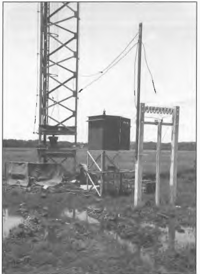
Nine wire unbalanced open wire transmission line of about 100 ohms impedance at 4QA Mackay together with aerial coupling unit and radiator base during installation 1957. The line wires were bridged to provide four active and five earthed conductors. Commissioning Engineer, Brian Robinson.
