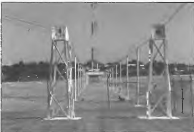
Dual 200 ohm 6 wire transmission lines at 5AN/5RN Pimpala NBS station erected 1961. Two 50 kW transmitters fed the dual frequency radiator.
