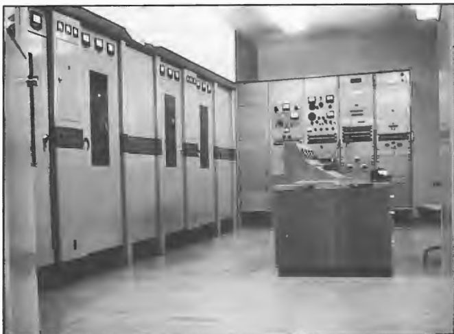
A pair of Philips 1656 transmitters manufactured in Adelaide and installed at 5DR Darwin 1955. The transmitters were originally installed at Gardens Hill but in 1965 were transferred to a new site at Ludmilla. They remained in service until 1978. Similar transmitters were installed at 5MV and 5PA in South Australia. Officer-in-Charge 5DR (changed to 8DR) was Ken Soar.
