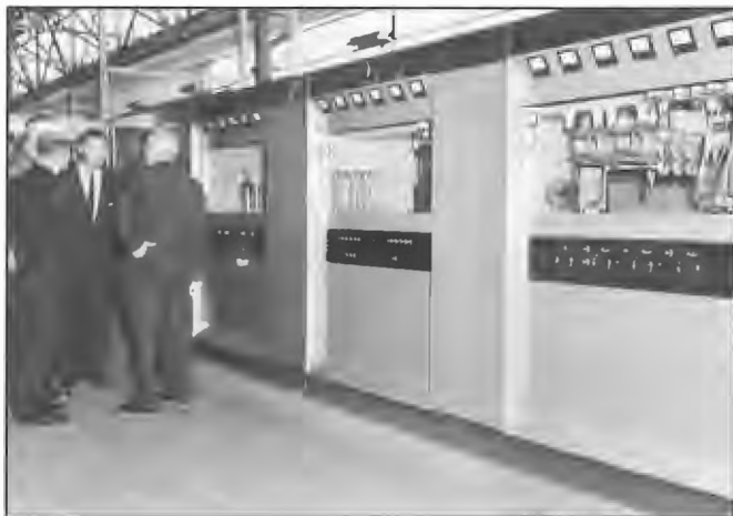
One of a number of 55 kW MF broadcast transmitters designed and manufactured by Standard Telephones and Cables Ltd in their Liverpool factory during 1950s-60s.
