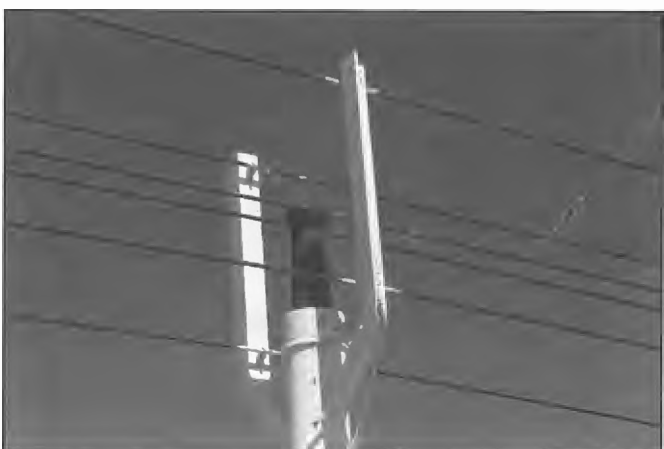
Typical six wire transmission line consisting of four earthed conductors and two central conductors attached to stand-off insulators. Characteristic impedance is approximately 200 ohms. One of the earliest lines to this design was provided at 2BL in 1942.
