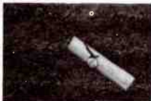
The ends of each loading coil are terminated as shown here. Heatshrink tubing is slipped over each coil and set in place to weatherproof them.
