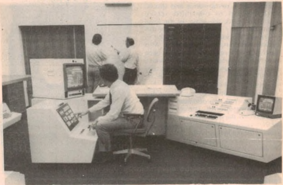
The control room of the Pipeline Authority's control centre at Young. Data is obtained from some 30 remote stations installed at intervals along the pipeline.
