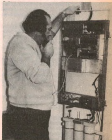
Doug Menneke, VK2ZMP, checking out the Wagga repeater at Mt. Flakeney during installation in June 1976.
