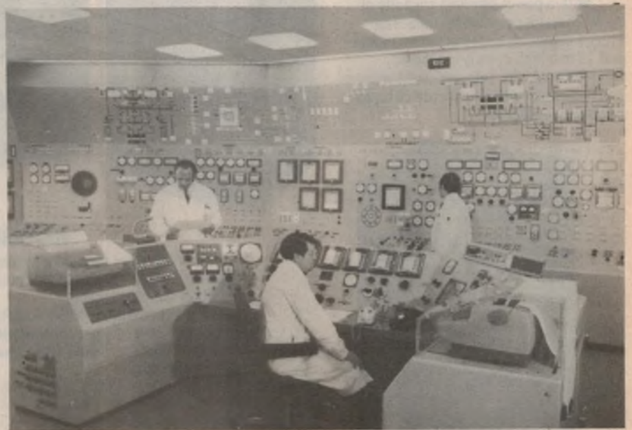
At top is an external view of the SGHWR at Winfrith while above is a view of the control room. The reactor was completed in 1967 and generates 100MW.
